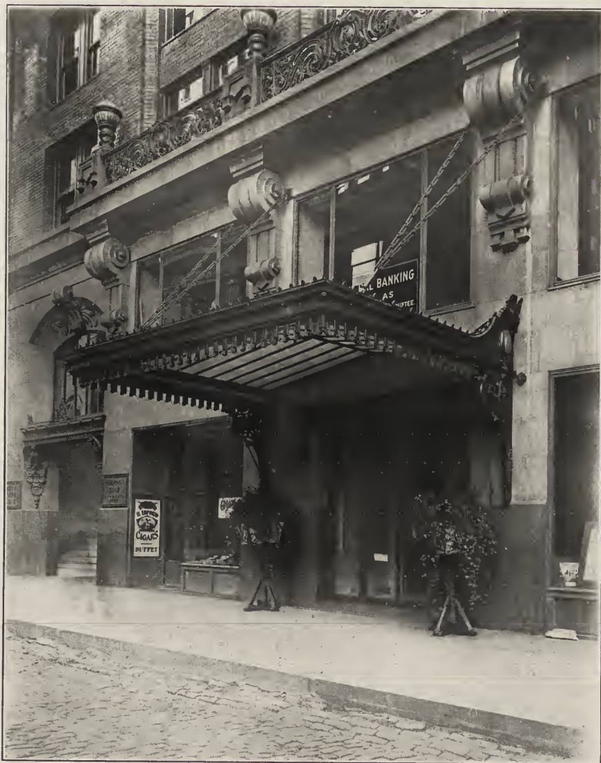
FIG. 7. A WELL-HUNG MARQUISE OF IRON AND WIRE GLASS. THE RECTOR BUILDING. Chicago, Ill.
