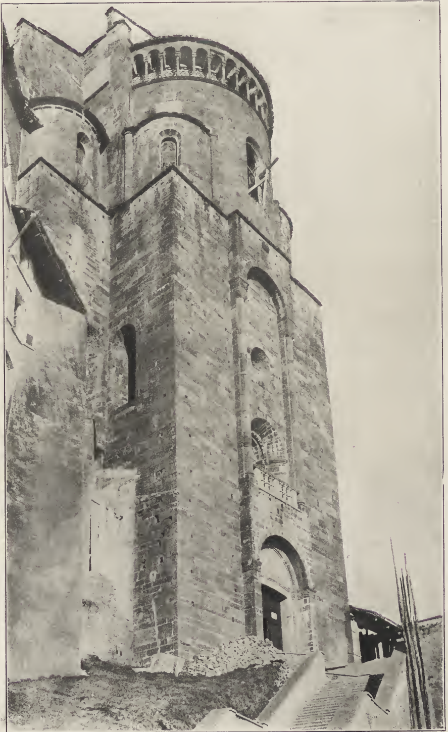
VIEW SHOWING THE MASSIVE WALLS SUPPORTING THE APSES OF THE SAGRA DE Piedmont, Italy. ST. MICHEL.
