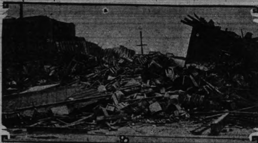
BUILDING COLLAPSES DURING FURIOUS STORM —During a storm, which swept from Illinois to Pennsylvania, the five-story brick building occupied by the Isaac Walker Hardware Company at Peoria, Ill., collapsed. Two men were killed when the building crushed a two-story garage next door.
