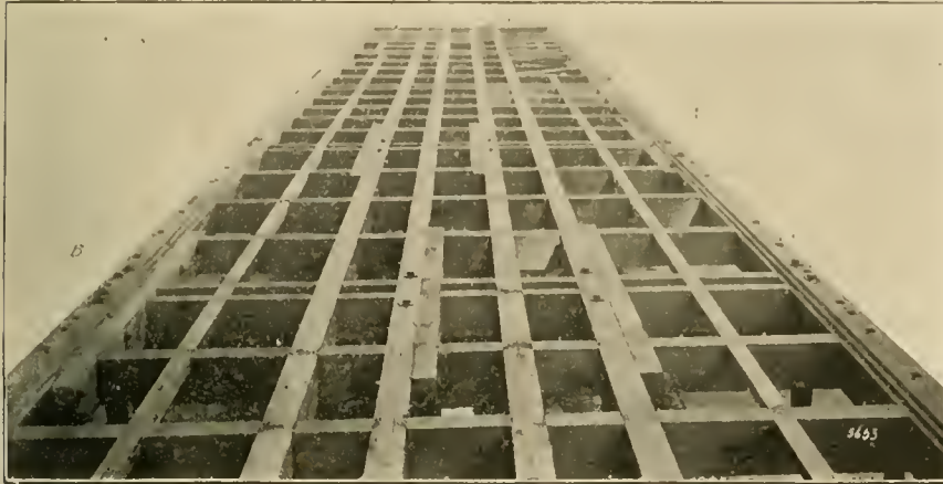
Spliced Passenger Car Sills.
