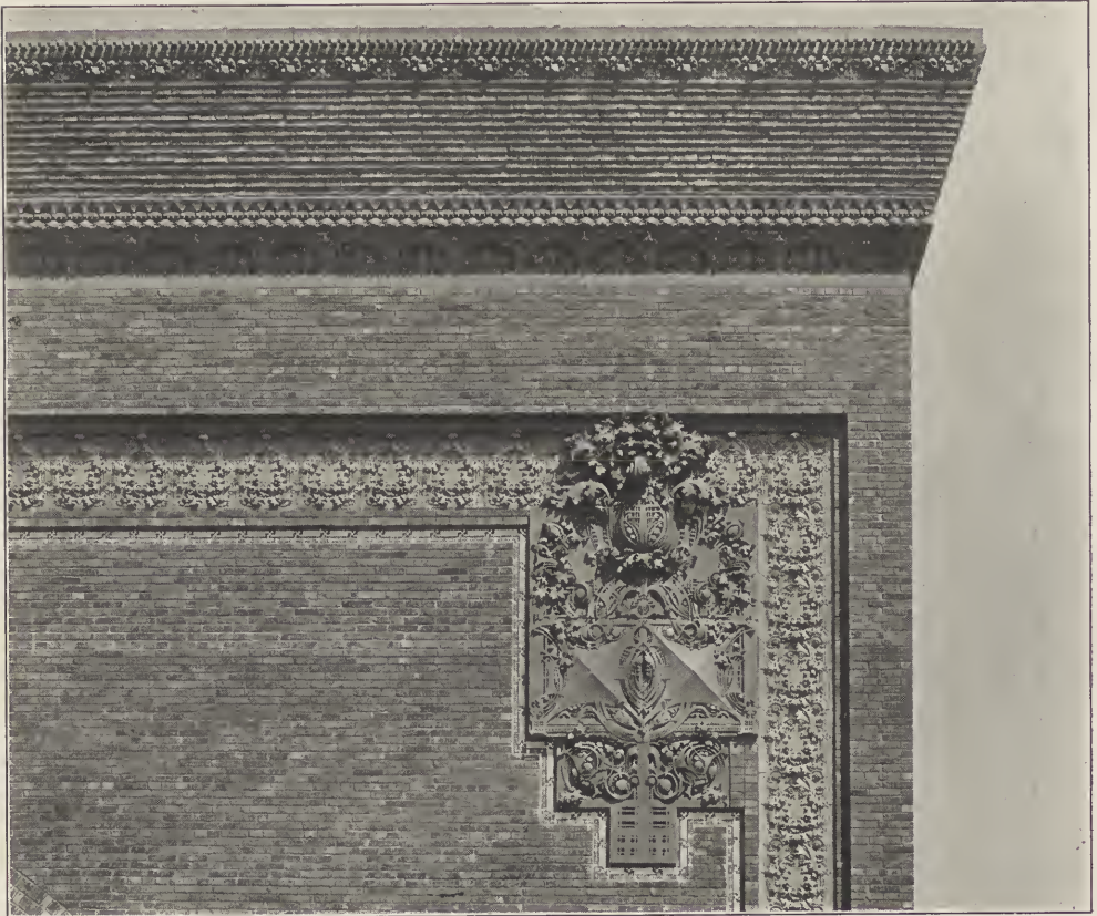
NATIONAL FARMERS' BANK OF OWATONNA, MINN.—DETAIL OF MAIN MASS. Louis H. Sullivan, Architect.
