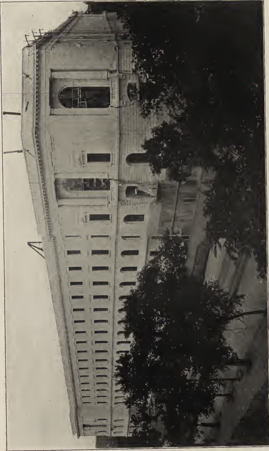
SENATE OFFICE BUILDING IN COURSE OF CONSTRUCTION—DELAWARE AVENUE AND B STREET FRONTS. John M. Carrère, Consulting Architect. Washington, D. C.
