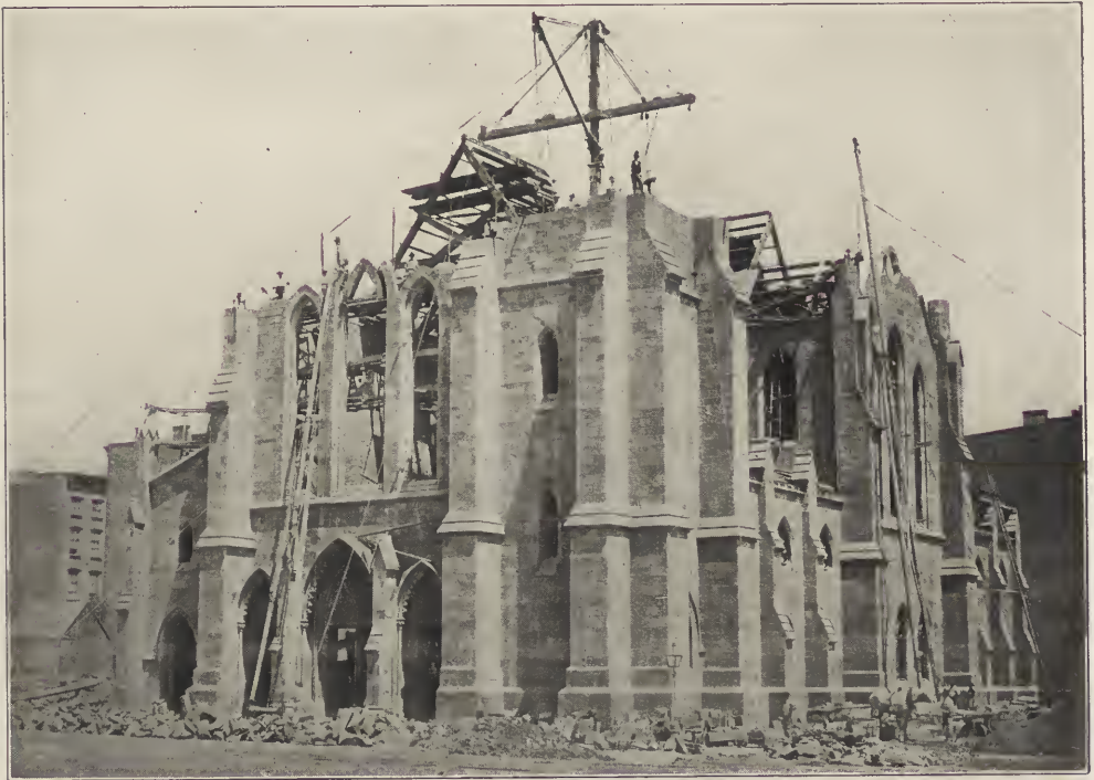
FIG. 9. THE BROADWAY TABERNACLE (1859-1905), DURING ERECTION. 6th Avenue and 34th Street, New York. Leopold Eidlitz, Architect.
