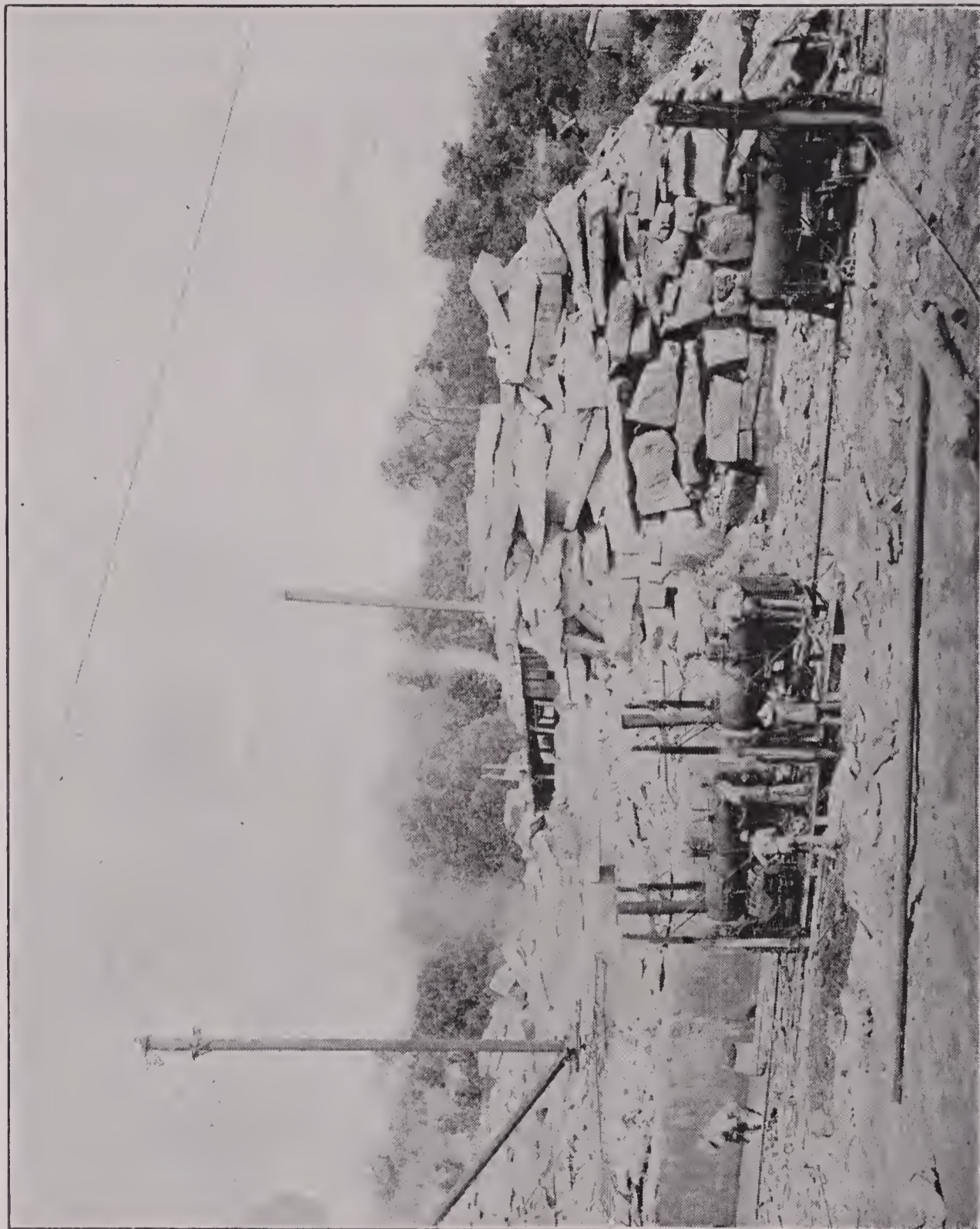
Fig. 26. An Oolitic (Salem) limestone quarry. The overburden which has been removed is Mitchell limestone. The first cut is being made in the upper surface of the Salem.
