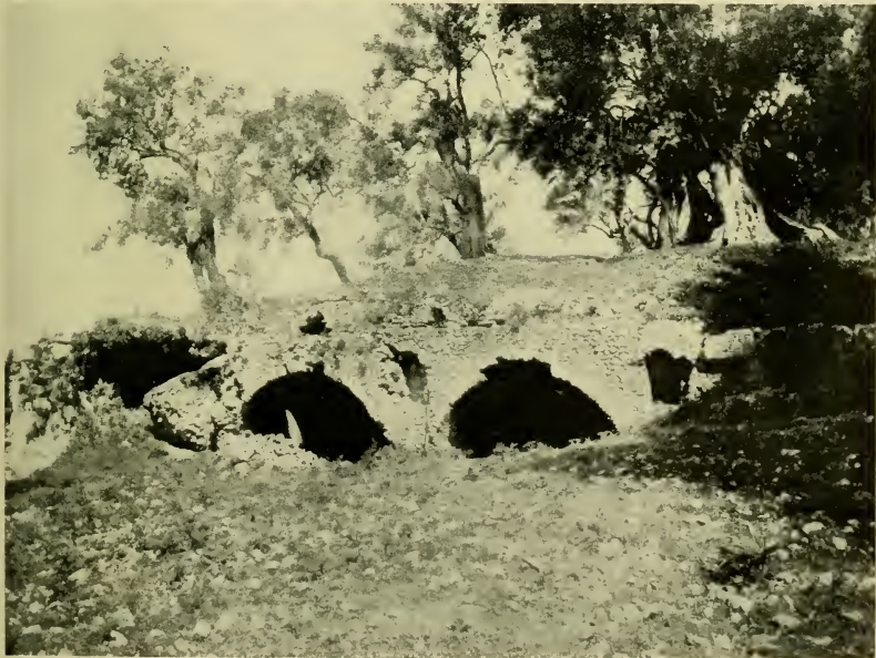
Sand and pebble catch-tanks on line of Marcia Aqueduct, near Tivoli. The catch-tanks are of small stone, Marcia of dimension stone
