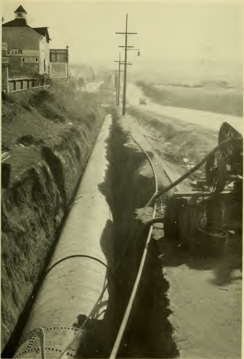
The fifty-four-inch San Andres line that will increase daily capacity from fifty to eighty million gallons
