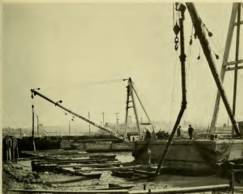
The submarine pipeline completely assembled and floated into place ready to be lowered, the end of the line being held in position by means of derrick barges.
