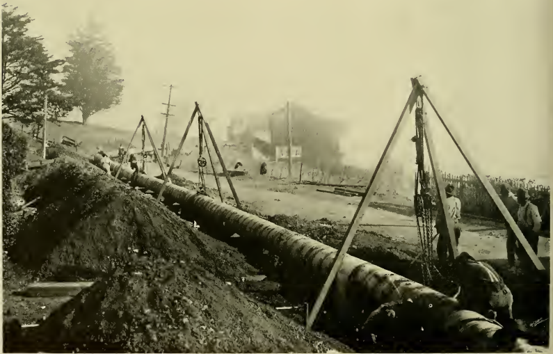
Spring Valley pipe crew installing a new line of twenty-four-inch riveted steel main in a district that has outgrown a smaller line. Pipe of this character is used for the larger distributing mains, cast-iron pipe being used for all lines tapped for house connections. Riveted iron pipe has lasted over fifty years in the streets of San Francisco.
