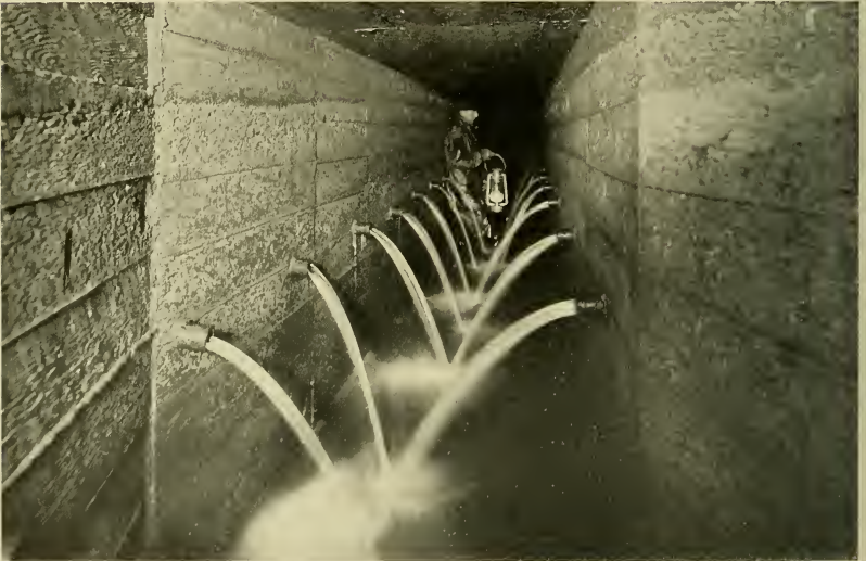
Beneath the floor of beautiful Sunol Valley are the infiltration galleries that gather the percolating waters of the gravel beds and deliver them to the Water Temple for the supply of San Francisco. This underground source is a natural reservoir and filter; the water is held back and forced into the galleries by Sunol Dam on Alameda Creek.
