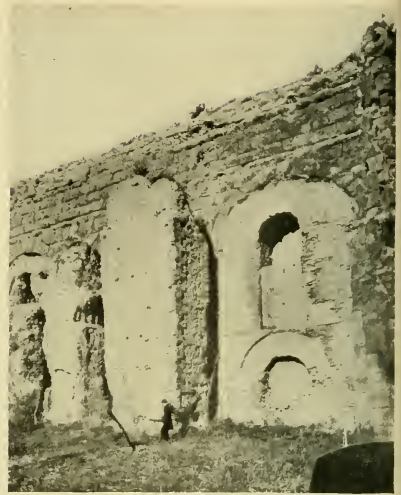
Claudia and Anio Novus near Porta Furba. Repairs were done in brick and in a composite of concrete and brick
