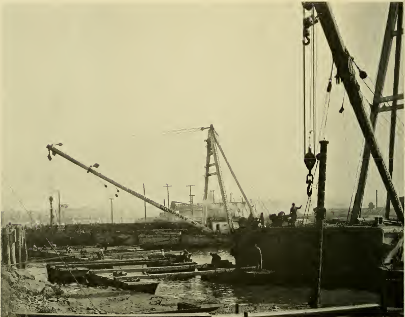
Lowering the main at Third Street and Islais. The men on the pontoons are handling the rope slings supporting the pipe. The entire installation called for unusual ingenuity.
