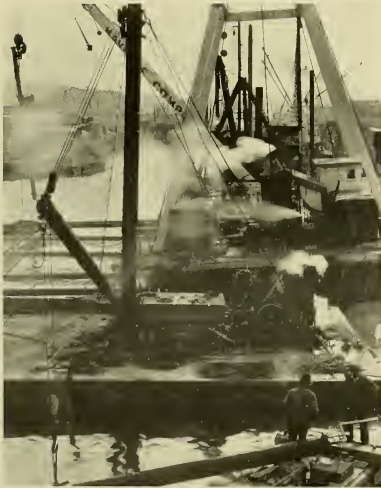
The pipeline at Fourth and Channel assembled on pontoons and ready to be moved into place.
