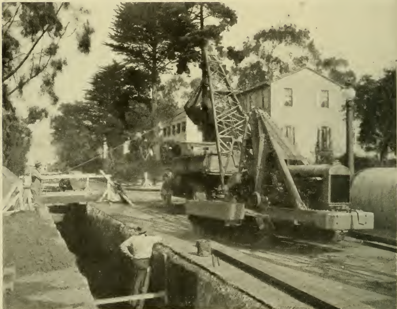
Great machines dig these trenches and quickly close them over the installed pipe
