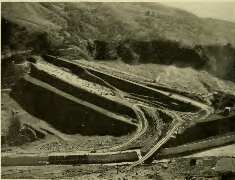
Calaveras Dam of Spring Valley Water Company carried to a height of 215 feet above its foundation. This view, like that on the cover of SAN FRANCISCO WATER , shows the berm construction of the down-stream slope
