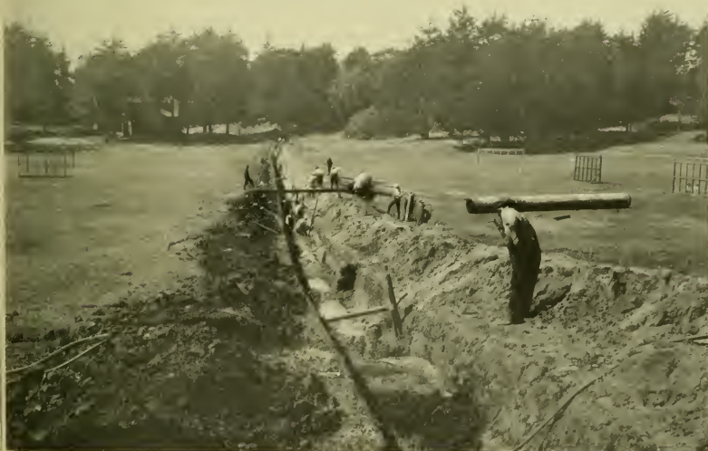
Above: Forty per cent of San Francisco will benefit by the new line from Laguna Honda. The new 36-inch steel main in Sixth Avenue looking toward Golden Gate Park, showing the bridges required for automobiles. Below: Crossing the baseball field in Golden Gate Park. Work was started on a Monday morning, and by the following Saturday noon the ball ground was again in use.
