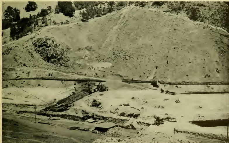
The white streak climbing up and down the hillside outlines the contact of the dam-to-be. This is a view of Calaveras dam-site looking east, before any fill was placed
