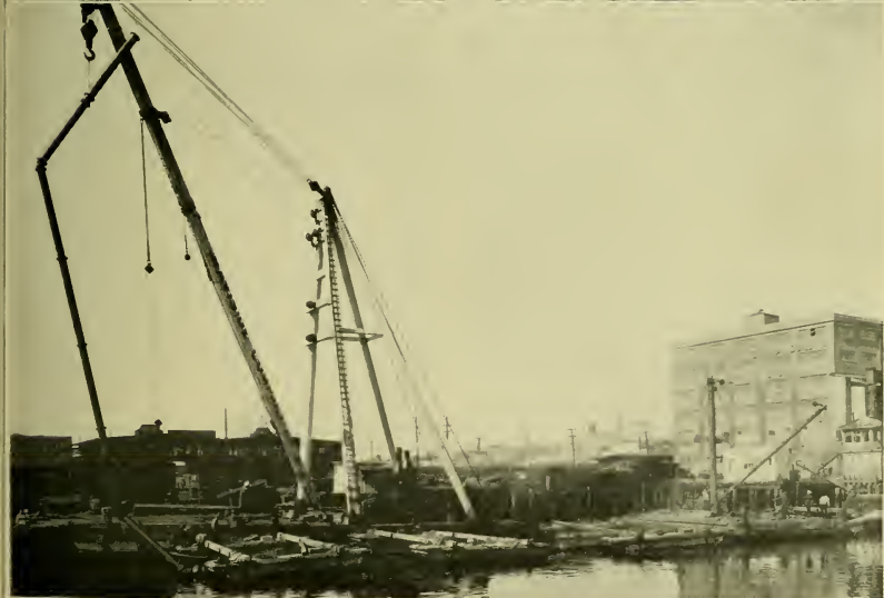
Here the camera records an unusual bit of water-supply installation—the laying of a submarine pipe across the Channel at Fourth Street, San Francisco. This pipe has flexible joints which enable it to accommodate itself to the uneven bottom. The length is 250 feet, and there are several angles. The pipe was put together on pontoons and lowered into place by derricks. The function of this pipe is to reinforce the water supply of the industrial district.
