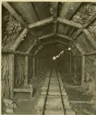
San Andres water will start toward San Francisco through this tunnel, eight feet high and eight feet wide
