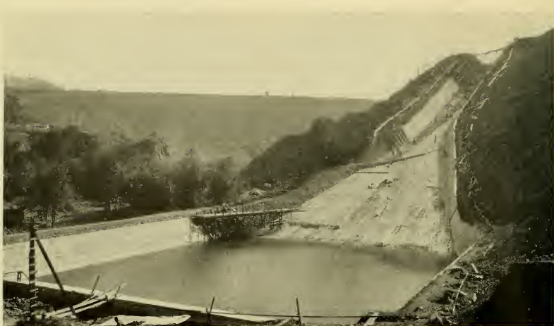
The spillway of Calaveras Dam is now completed. It had reached the above stage of construction in September, 1924. The top of the dam is seen on the skyline
