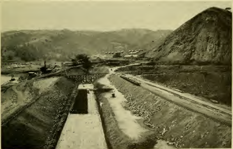
Rolled clay core of Calaveras Dam under construction. This core, which is supported by the embankments of rocky material, is now completed to a height of 215 feet
