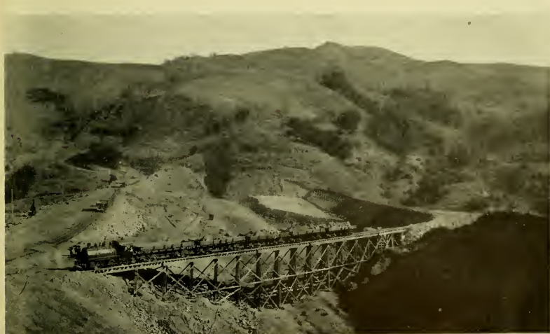
Calaveras Dam becomes a part of the landscape. There were 2,312,000 cubic yards of material in place when this view was taken in January, 1924
