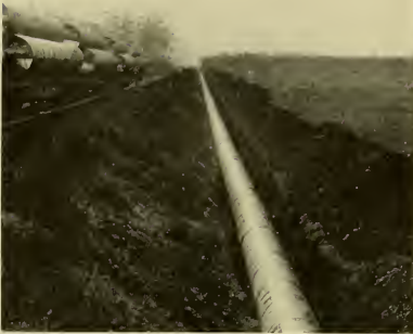
Spring Valley's Niles-to-Irvington forty-four-inch pipe-line will carry Calaveras water to the Irvington inlet of the Hetch-Hetchy Conduit, through which the water will flow to Crystal Springs Reservoir in San Mateo County. The pipe on the car has since been laid
