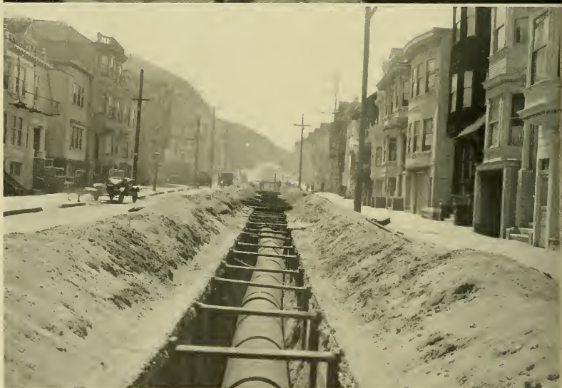
Above: Installing a new line from Laguna Honda Reservoir. A twenty-inch connection at Sixth Avenue and Lincoln Way between the twenty-four-inch cast iron and the new thirty-inch steel main, looking toward Golden Gate Park. Below: The new 36-inch steel main in Sixth Avenue, in the Sunset District, placed in the trench ready to be welded. Due to the sub-soil being sand, every foot of the trench had to be supported as shown.
