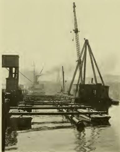
Assembling the 12" cast-iron main on the pontoons along-side of the wharf on Islais Creek at Third Street.
