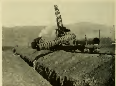
Laying pipe for Spring Valley's Niles-to-Irvington Line. By using the caterpillar crane, the two operations of unloading cars and placing pipe in trench are combined in one
