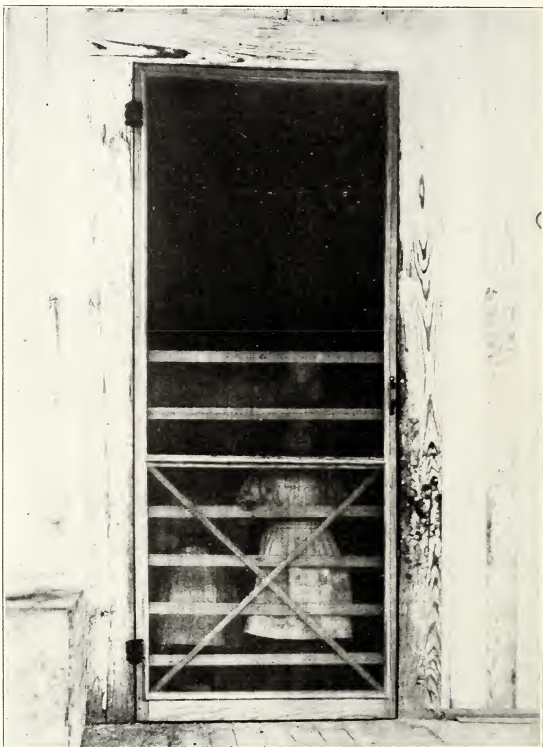
FIG. 27.—TYPE OF DOOR SCREENING INSTALLED, HOUSES OF GROUPS "A" AND "C."
