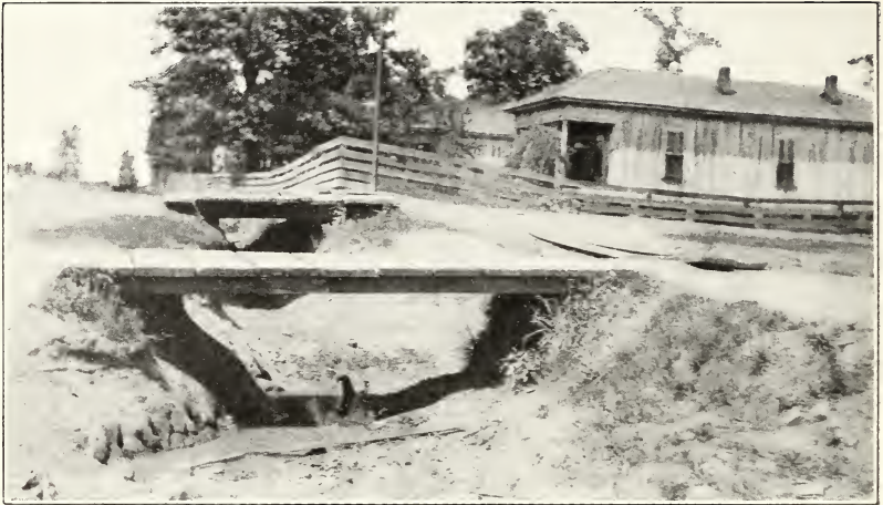
FIG. 11.—STREAM "E," "COLORED TOWN," CROSSETT, SHOWING "POT HOLES."
