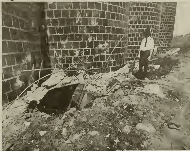
EAST END OF TUNNELS BENEATH TANKS Note the violence of explosion, as shown by manner in which concrete reinforcements were blown out
