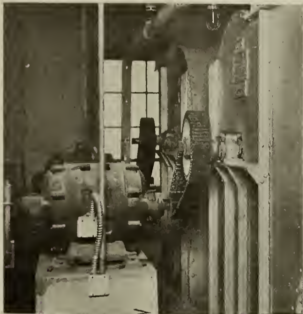
Morse Drives on Elevator Legs
