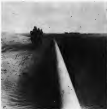
A World Bank loan helped finance this 16-inch, 350-mile long gas pipeline from the Sui field in Baluchistan to Karachi
