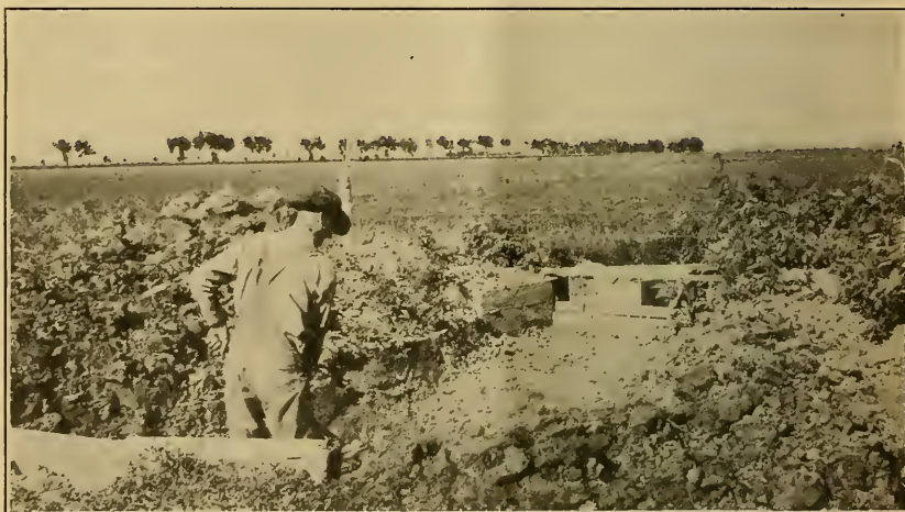
FIG. 9.—Removing silt from an irrigation ditch. In order to insure rapid delivery of water when the crop requires it, some work must be devoted to cleaning ditches a few weeks prior to the first run in the canal.
