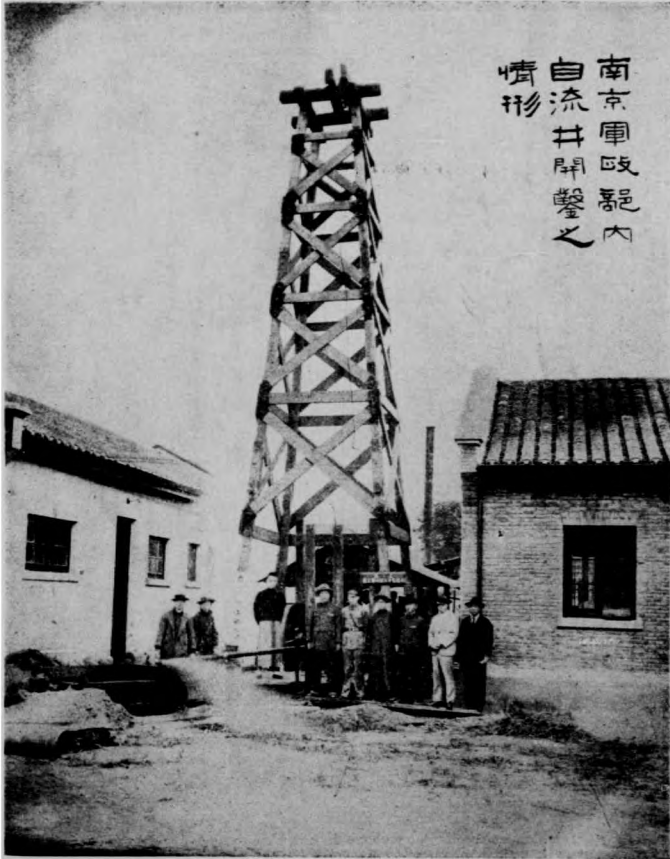
南京三牌樓軍政內部自流井開鑿之情形 Well drilled by Ministry of Military Affairs at San Pai Lou, Nanking.
