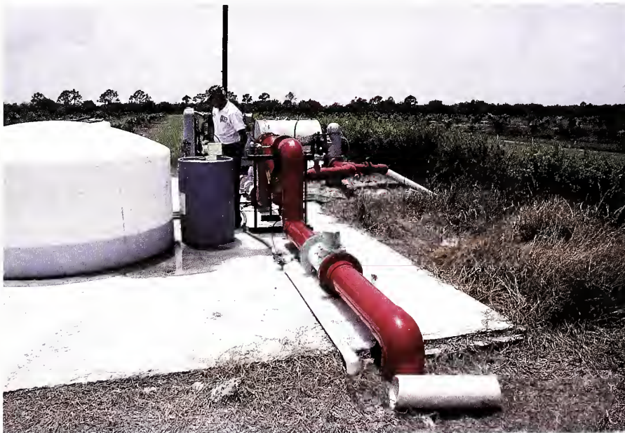
Keeping pumps efficient through maintenance saves fuel and water and ensures the uniform delivery of water and the fertilizer that is often mixed with it. (Art Greenberg photo; 0792-08)
