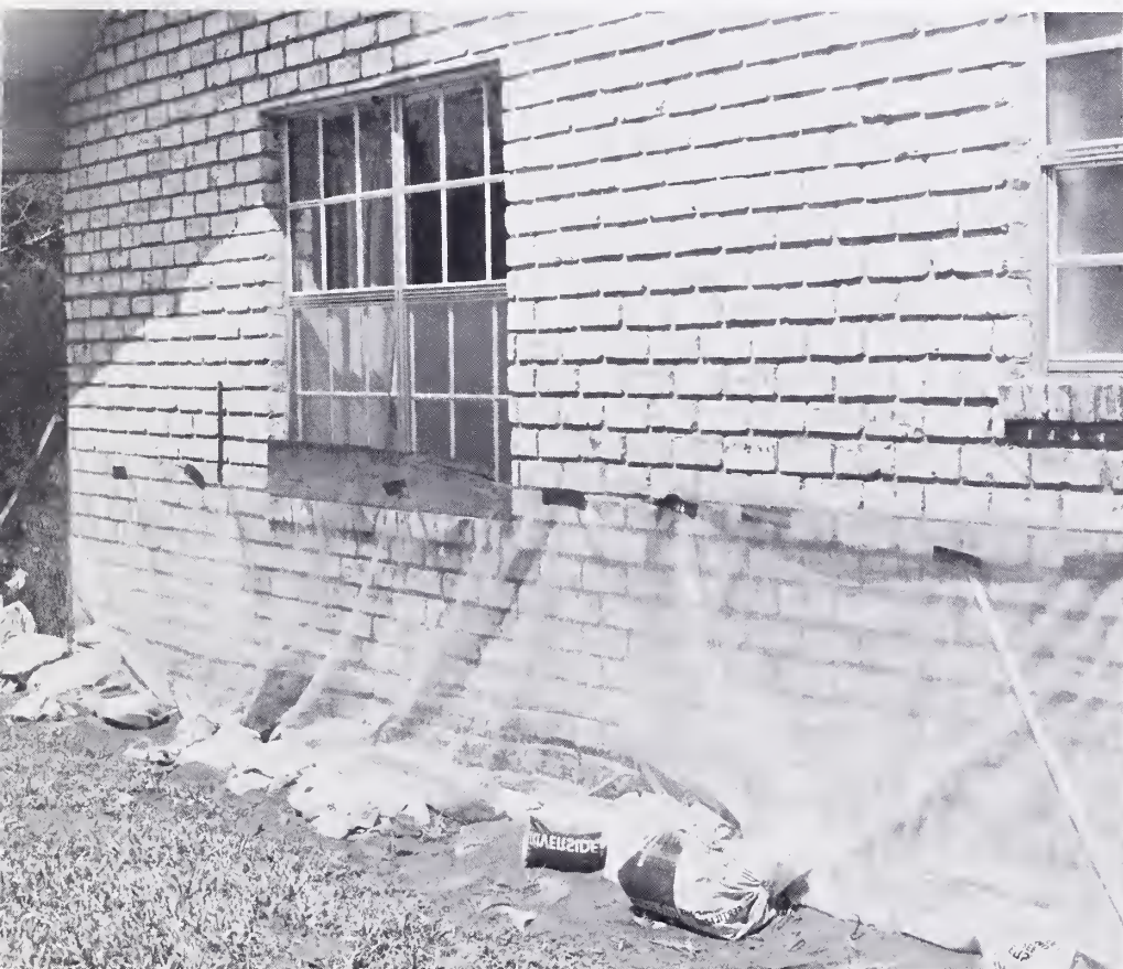
The polyethylene plastic sheeting around the McManus home was attached to the outside walls with masonry nails.
