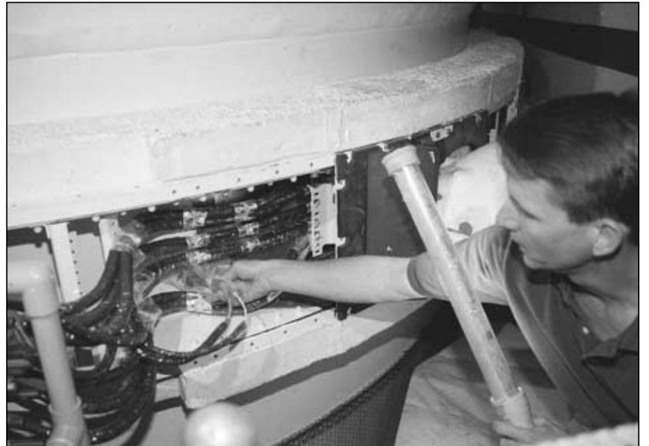
A KSC worker inspects the reusable cable and connectors located inside the external tank attachment ring on Atlantis ' left-hand solid rocket booster in December.
