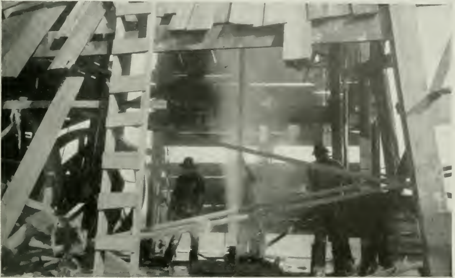
Swinging a length of 3-inch tubing to place over the high pressure gas flow.
