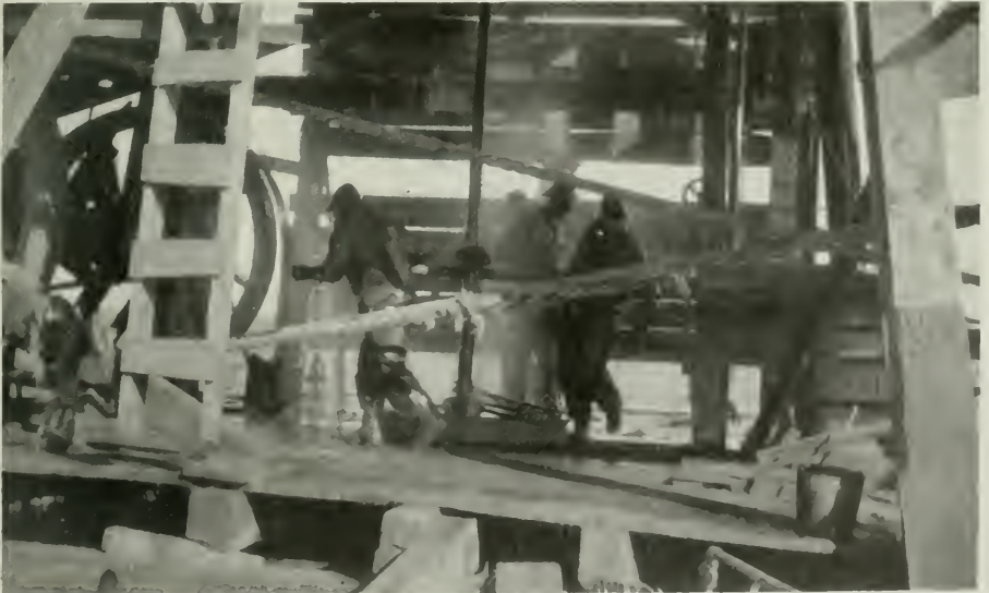
"Bucking up" the tubing. "No sleep until the well is closed in."
