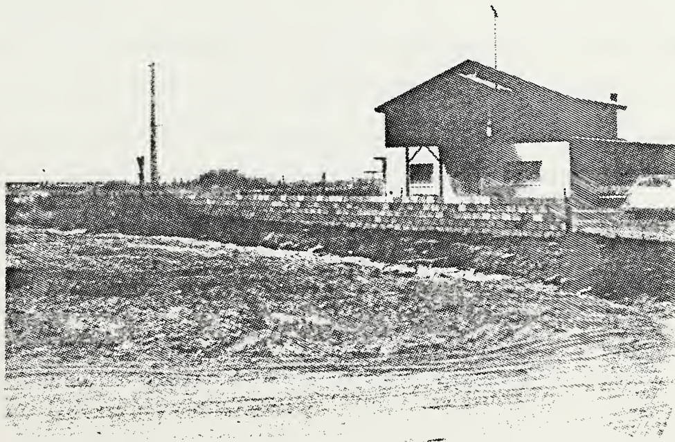
Figure 8 Flood Proofing of House North of and Adjacent to School House Wash
