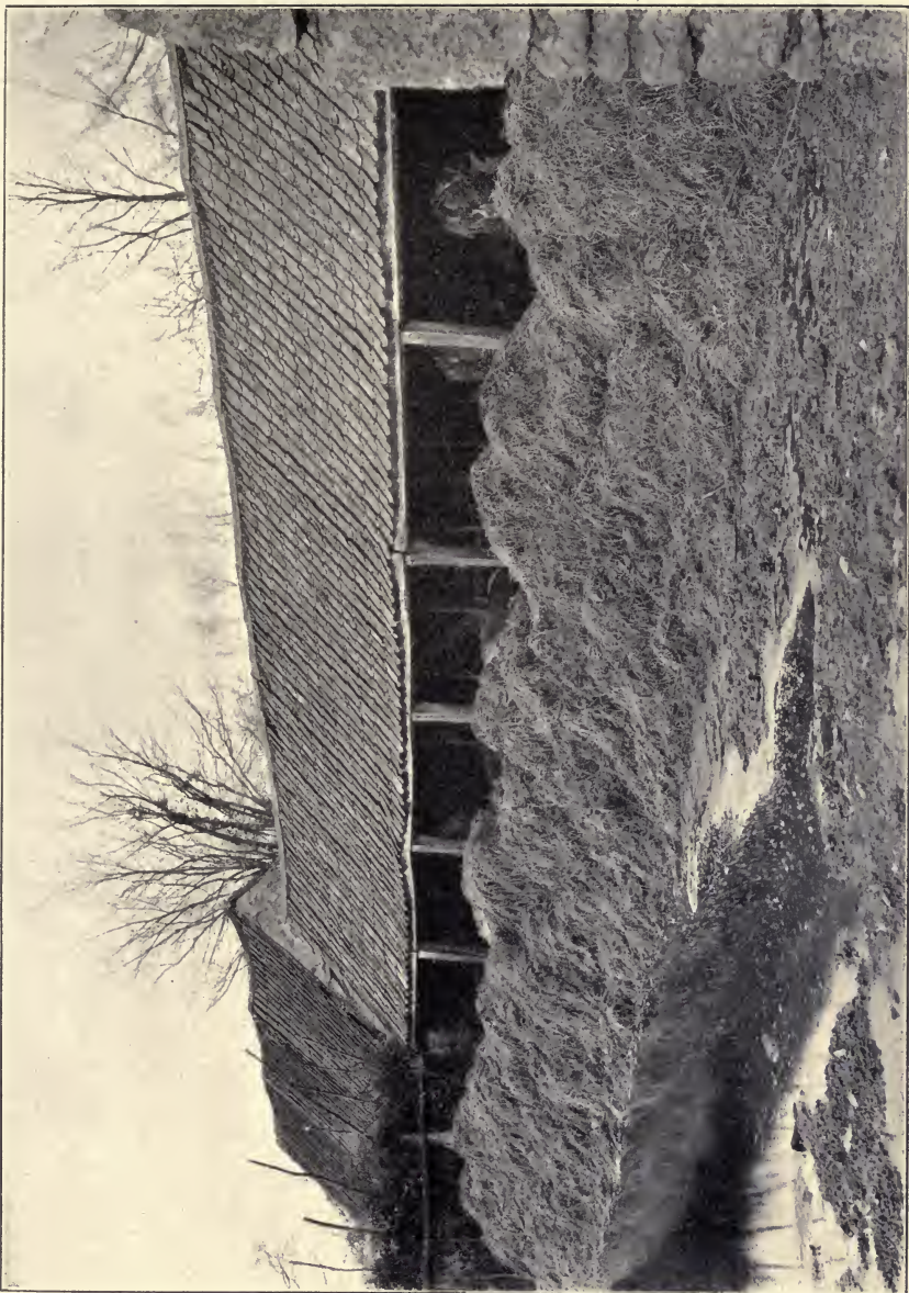
FIG. 15.—Immense Wall of Manure just outside Shed and a foul pool of Yard Drainage and Manure Soakage; cows milked in the shed.
