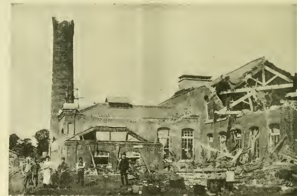
FIG. 2.—Nagoya Spinning Mill. Showing the effects of the Mino-Owari Earthquake of 1901 on a brick building and on a chimney constructed according to European practice.
