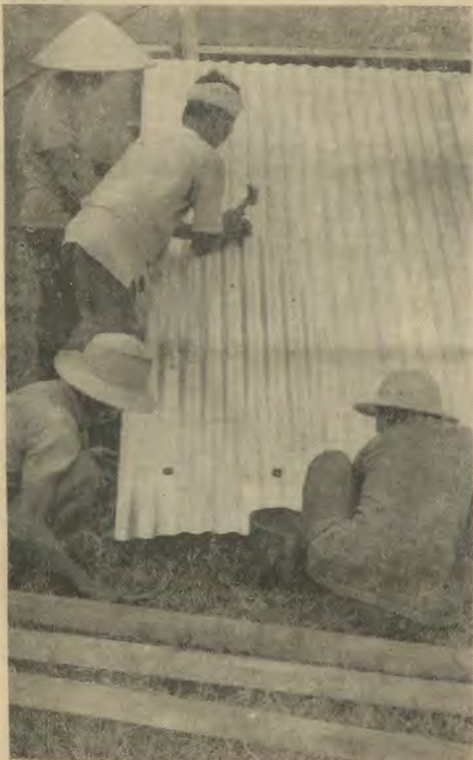
TIN ROOF — USAID supplied materials in the hands of men with a community spirit will provide for the homeless at Dia Loc
