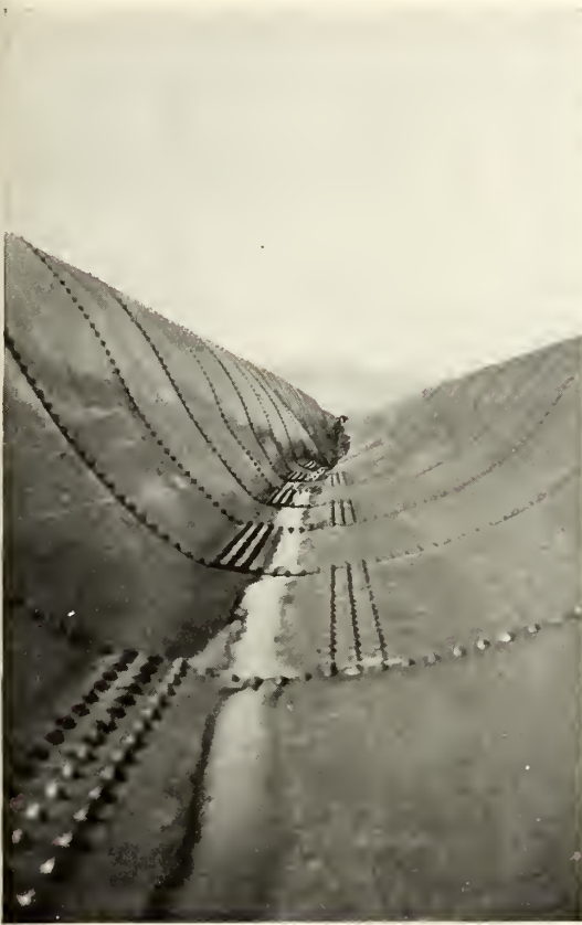
THE COLLAPSED SIPHON. (SEE PAGE 348.)
