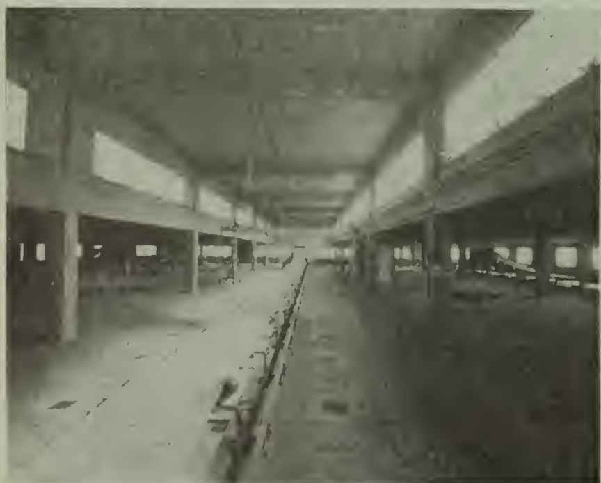
One of the belt conveyors in the new Murray Elevator at Kansas City, Mo., which is served by 2,000 feet of SUPER-SERVICE Rubber Belting.
