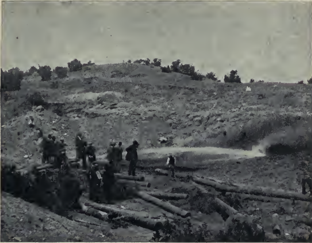
A. BUILDING DAM BY HYDRAULIC PROCESS AT SANTA FÉ, NEW MEXICO, SHOWING HYDRAULIC GIANT IN USE.
