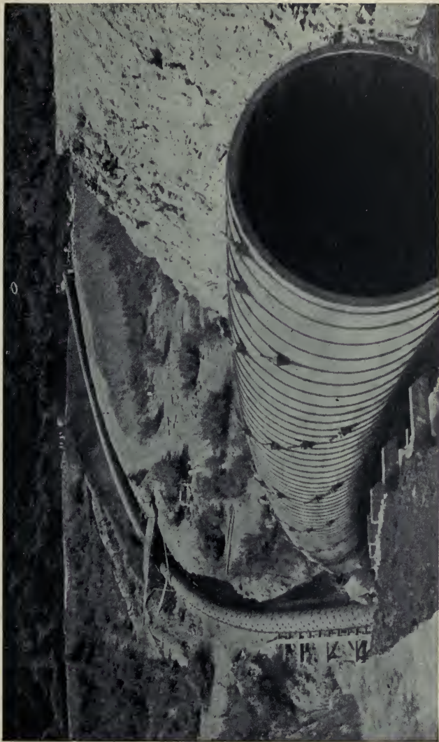
REDWOOD STAVE PIPE 52 INCHES IN DIAMETER CROSSING WARMSPRINGS CANYON, NEAR REDLANDS, CALIFORNIA.
