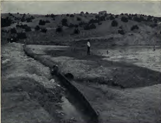
B. BUILDING DAM BY HYDRAULIC PROCESS AT SANTA FÉ, NEW MEXICO, SHOWING OUTLET PIPE.
