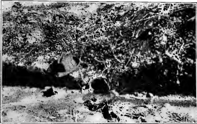
FIG. 29. — Drainage outlet that is likely to clog.
