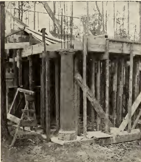
FIG. 1. A CORNER OF A "REINFORCED" CONCRETE HOUSE IN PROCESS OF CONSTRUCTION. NOTICE THE IRON RODS PROJECTING FROM THE CEMENT COLUMN AT THE CORNER.
