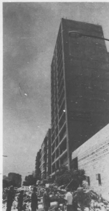
Office building leans forward. U.S. Trade Center is at lower right. (Photo by Tomas Moreno Arreola)
