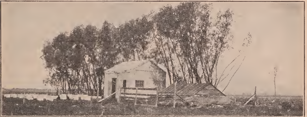
Fig. 6.—E. G. Brown's upground cellar constructed by setting four fence posts about four feet into ground at the four corners of the proposed cellar. The portion of the posts above ground are boarded up on the outside. The dirt on the inside is shoveled out, forming an embankment around the board fence. The whole is covered with a roof as shown.
