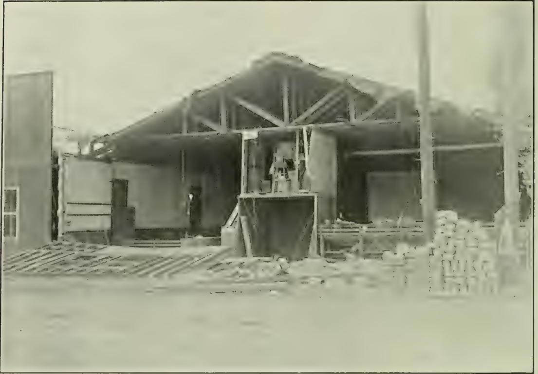
FIG. 1. A MOVING-PICTURE THEATER AT SAN JACINTO, CALIFORNIA, AFTER ITS FRONT WALL HAD FALLEN TO THE STREET DURING A RECENT EARTHQUAKE. The concrete-block type of construction is dangerous in a region of high seismicity. (Photograph by S. D. Townley.)
