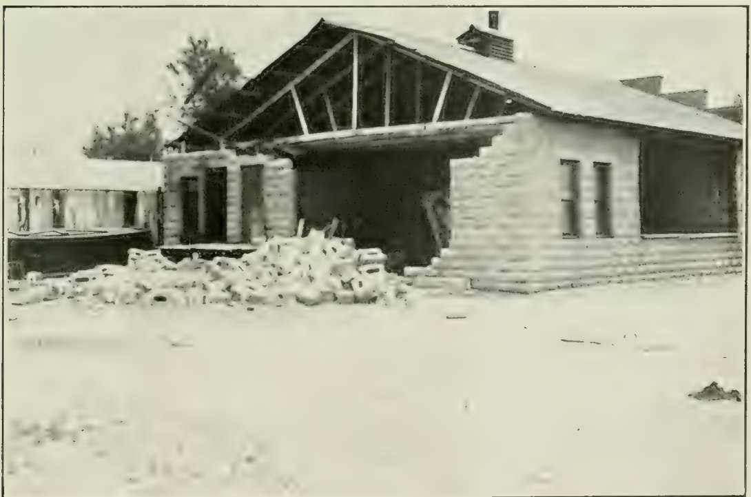
FIG. 16. A CONCRETE-BLOCK BUILDING WRECKED BY AN EARTHQUAKE. Experience has shown that reinforced concrete, steel-frame and wooden buildings will stand through severe earthquakes, whereas brick, concrete-block and adobe buildings are easily destroyed. (Photograph by Homer Hamlin.)
