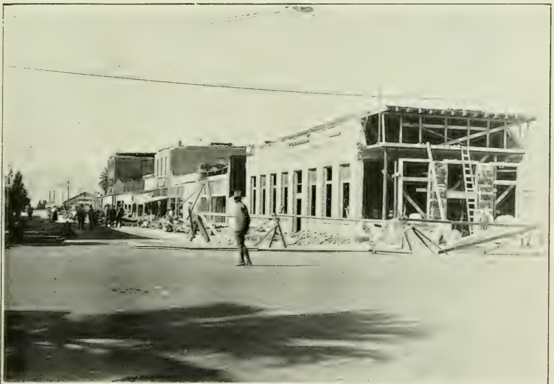
FIG. 6. A VIEW OF THE FIRST NATIONAL BANK BUILDING AT HEMET, CALIFORNIA, JUST AFTER THE EARTHQUAKE OF APRIL 21, 1918. (Photograph by S. D. Townley.)
