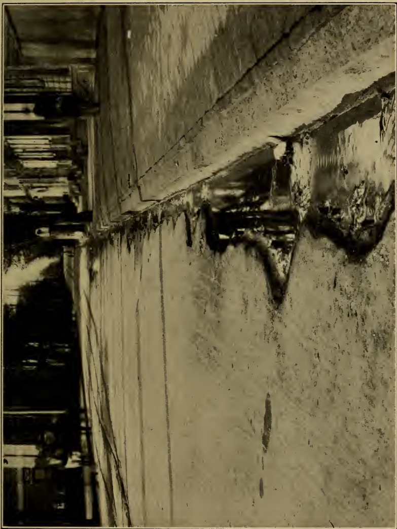
FIG. 19.—Bermudez Asphalt Surface Disintegrated by Water.
