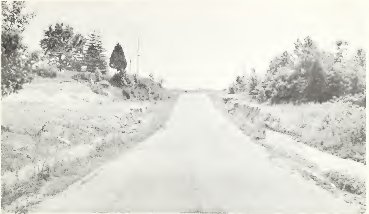
Typical roadbank sediment producing area.
