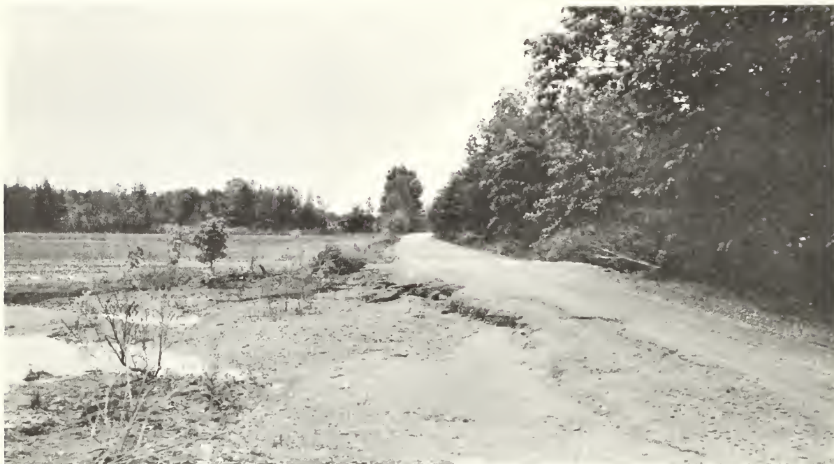
A typical scene of floodwater damage to county roads within the watershed. Note gravel deposit in field at left.
