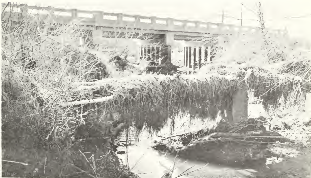
Drift collection on sewer and water pipelines on Crooked Creek above Federal Highway 45 just south of Selmer. During the April 1963 flood, floodwaters covered this road due to inadequate capacity under bridge.
