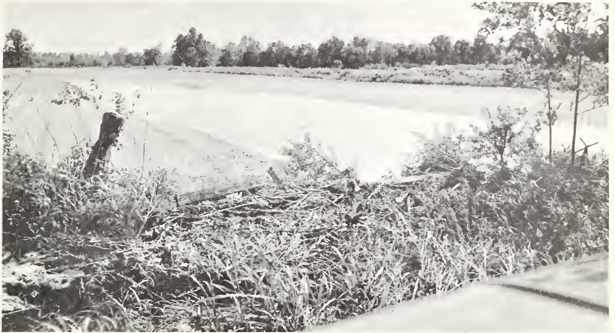
Typical fence damage. Note how fence has been completely destroyed due to the collection of drifts.
