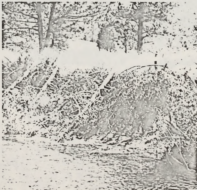
Figure 6 After. Junipers were placed on the bare, eroded bank during the summer of 1977. This photo was taken during the fall of 1978. Banks have sloped due to silt deposition and the establishment of riparian vegetation.
