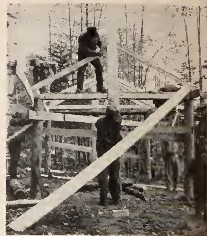
Volunteers construct a picnic shelter as part of Washington County's development of recreational resources.
