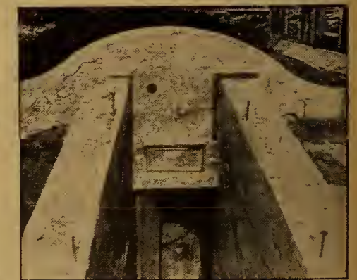
Entrance before door frame and door were put in place. The cave is nine feet deep
