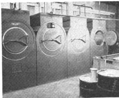
A scene in a typical dry cleaning plant showing the exhaust ducts for drying tumblers. Photograph courtesy of Pennsylvania Department of Health, Bureau of Industrial Hygiene.
