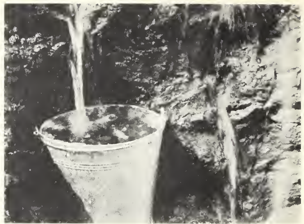
Figure 47. Snowmelt water discharging from road cut 10 feet below ground surface. June 16, 1950.
