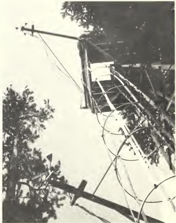
Figure 114. Looking up at middle and top anemometers on windtower in forest.
