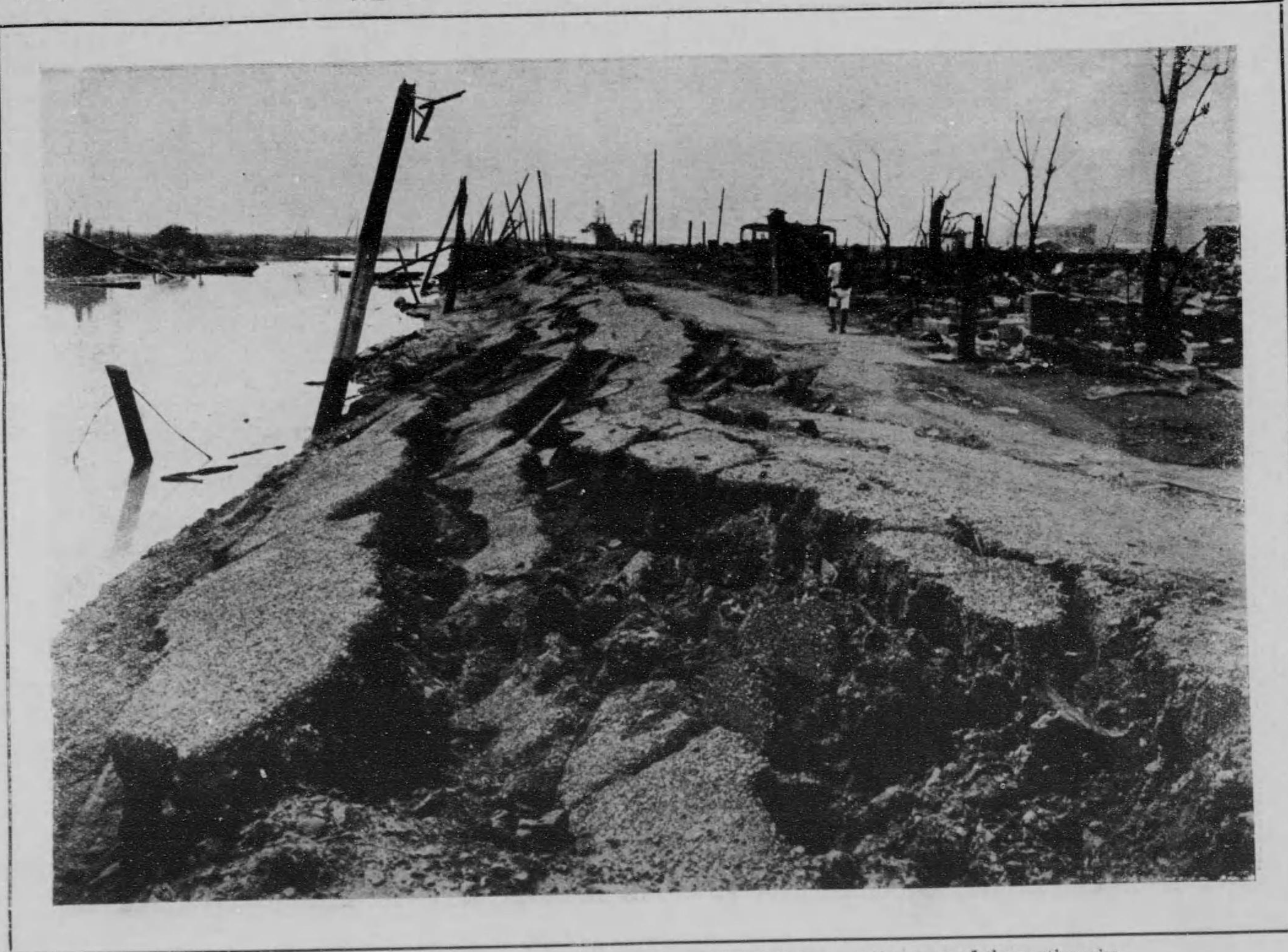
Fissures on the street at Kumoi-cho, Yokohama. A sample of the tremendousness of the earthquake.
