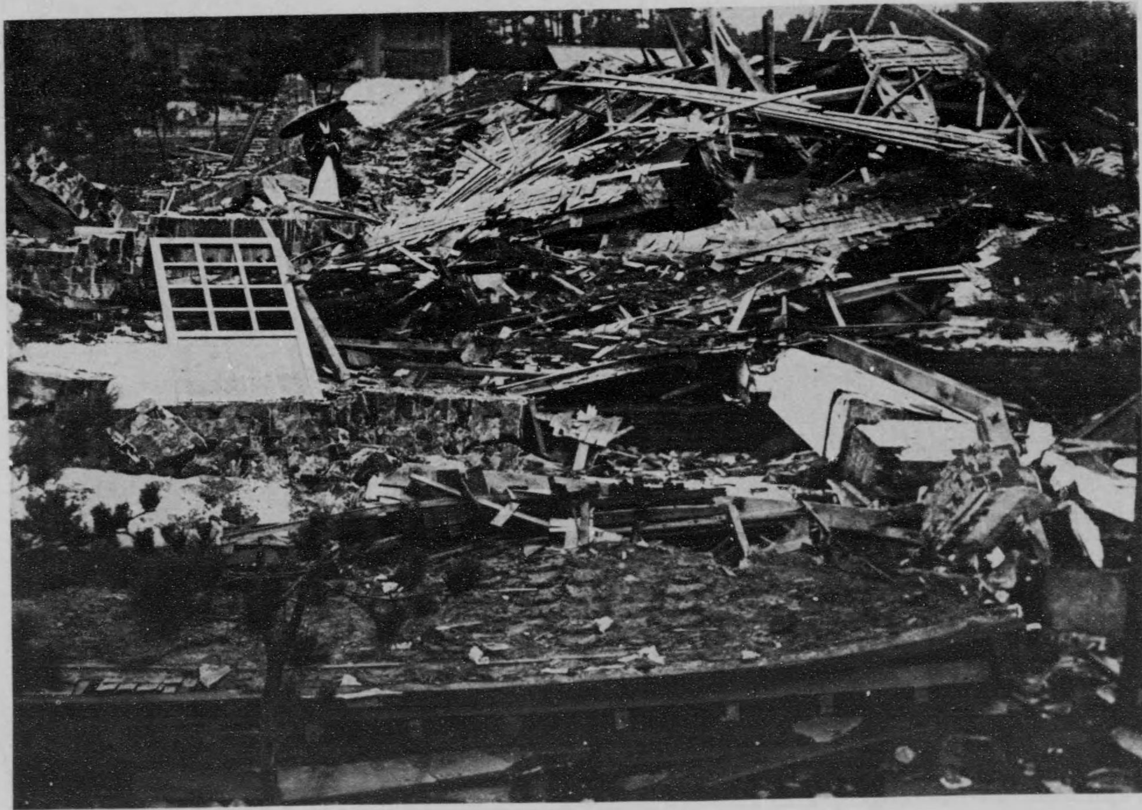
Damages of Sojiji, a grand temple of the Sodoshu sect at Tsurumi near Yokohama. Left: Ihaido, the hall of ancestral tablets, completely collapsed.
