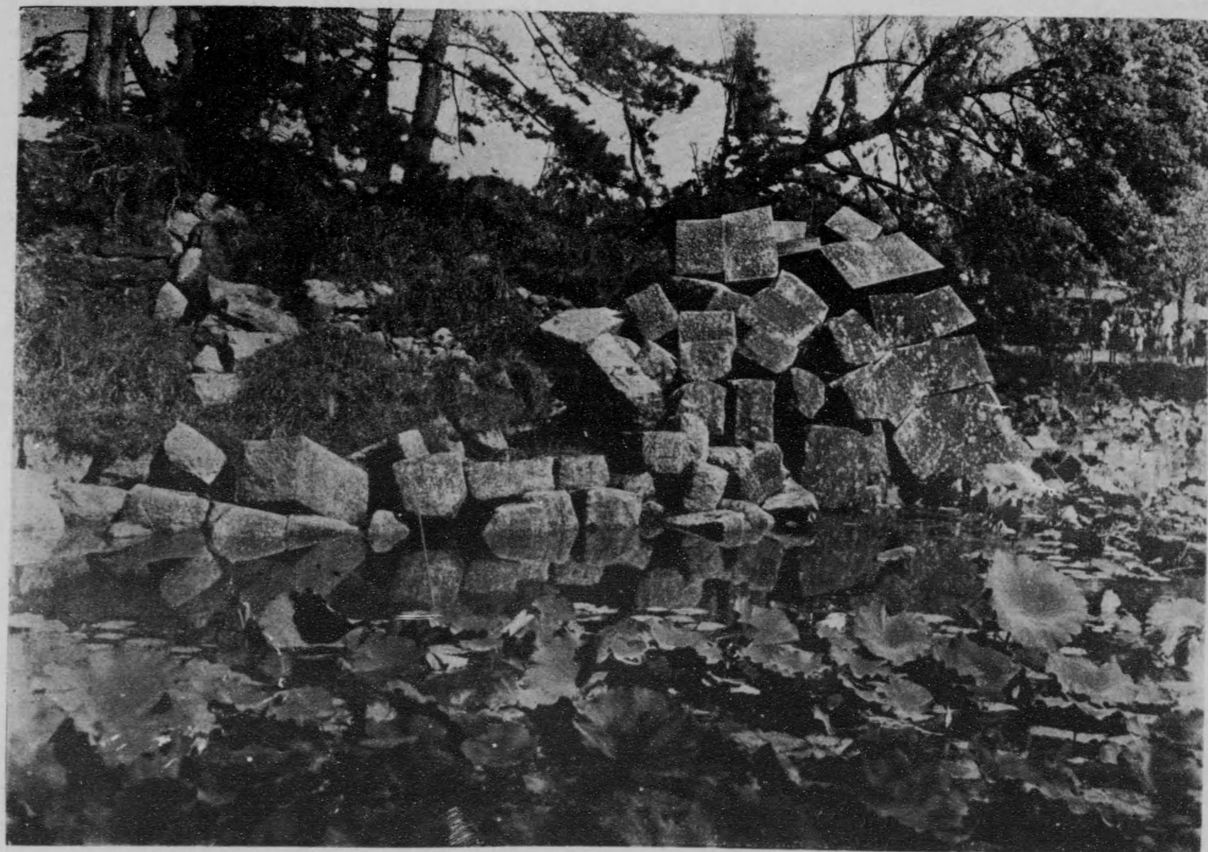
Broken wall of the Odawara Castle.
