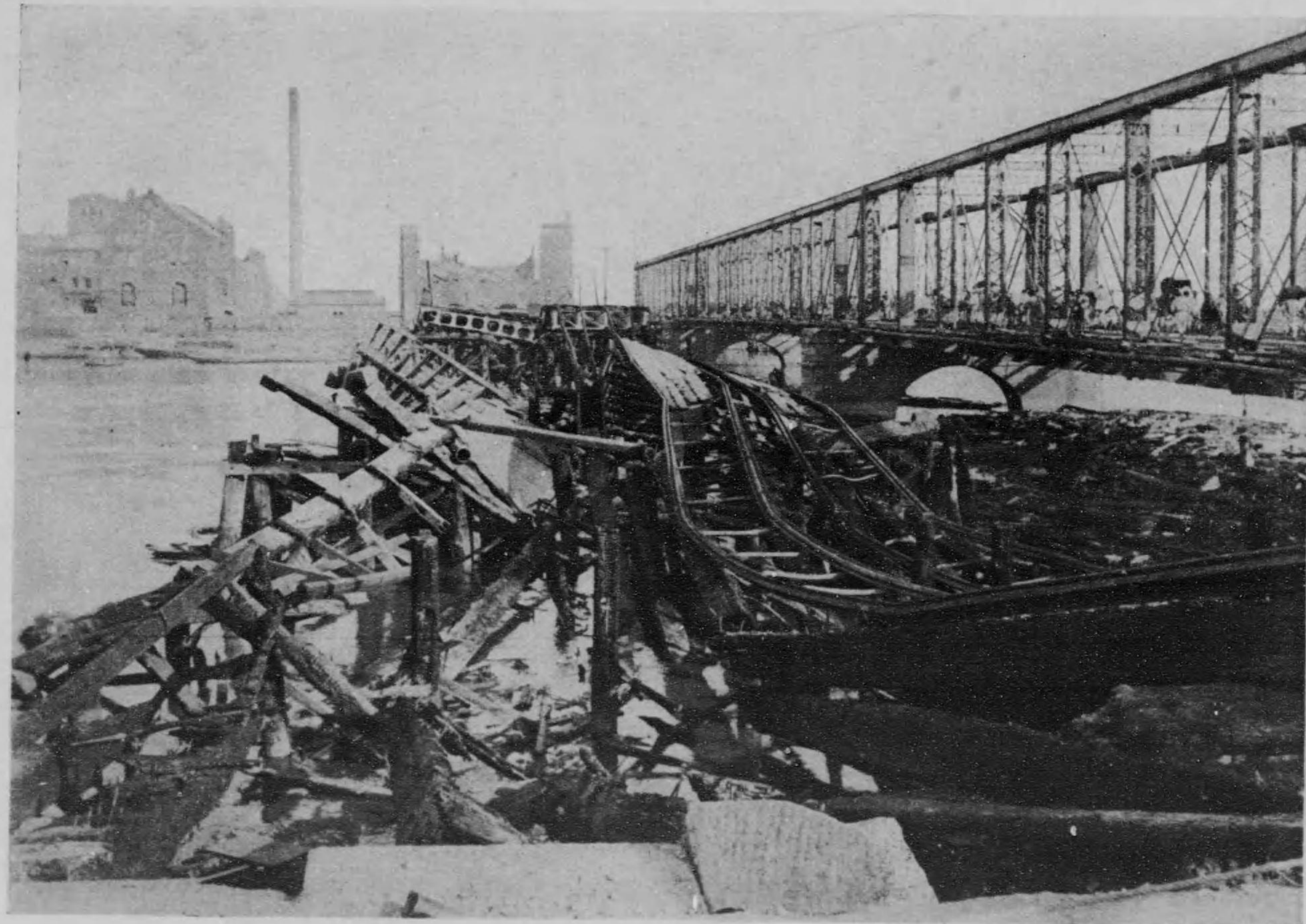
Azuma-bashi Bridge, which was under reconotruction was burnt down together with a temporary bridge span for the purpose.
