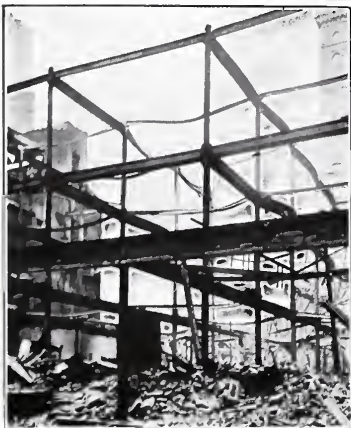
Keystone Cast Iron Columns Intact After a Big Pittsburgh Fire
