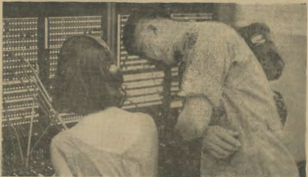
VUNG TAU SWITCHBOARD — Sergeant First Class Felix Canyon, of Pearl City, Hawaii, NCOIC of the Vung Tau switchboard, assists a Vietnamese operator in getting a telephone call through for a subscriber.
