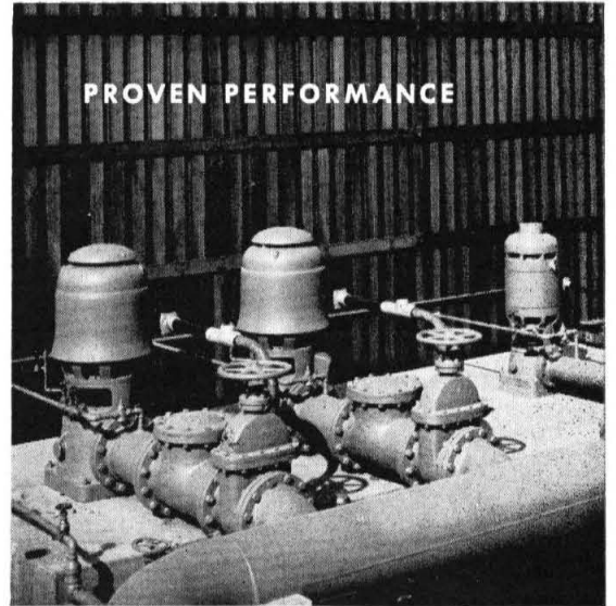
Three of fourteen pumps installed in a prominent Southern California aircraft plant. Circulating cooled water is one of many industrial applications for Wintroath Pumps.
