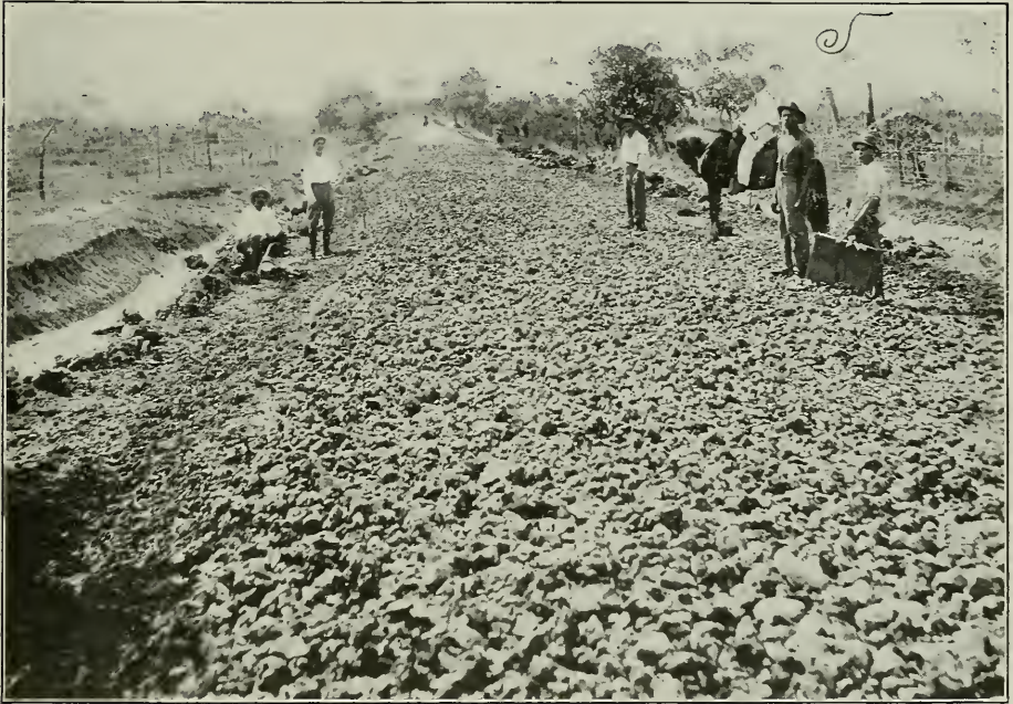
Road from Puerto de Golpe to Pilotos under construction—Pinar del Rio Province.
