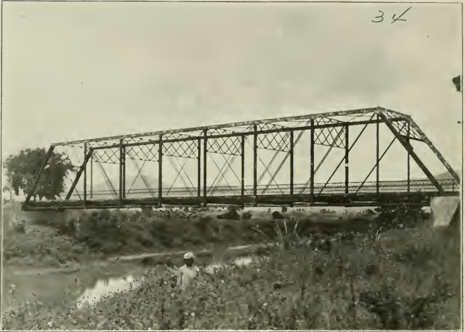
Bridge over San Cristobal River along the Central Road after repairs— Pinar del Rio Province.
