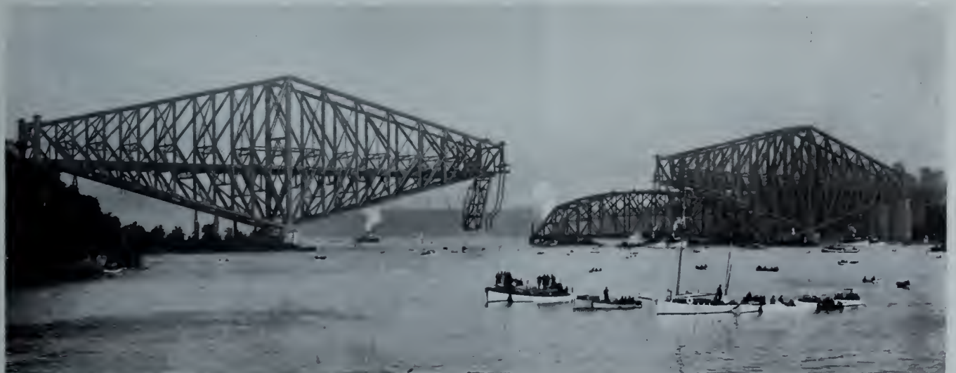
PONTOONS WITH CENTRE SPAN ABOARD BEING MOVED INTO POSITION FOR LIFTING OPERATION.
