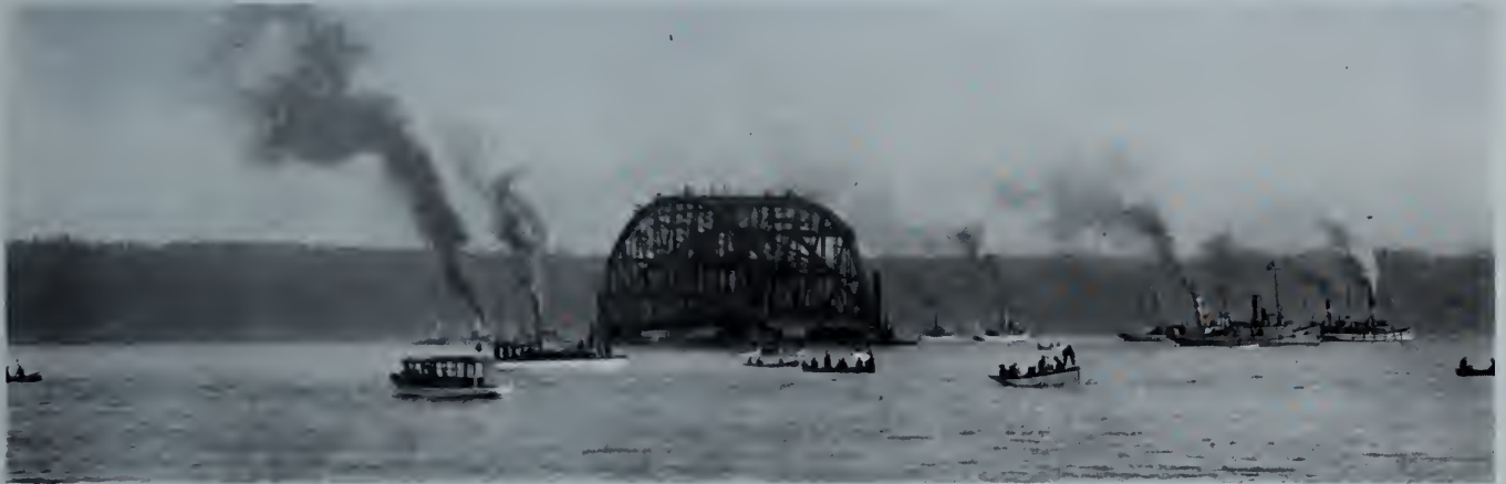
PONTOONS WITH CENTRE SPAN ABOARD BEING TOWED FROM SILLERY COVE TO THE BRIDGE SITE.
