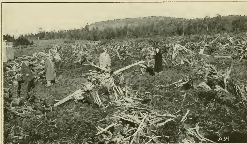
The sort of wreckage practically perfect stump blasting should give. The pieces are shattered so they are easy to handle and so they burn well.
