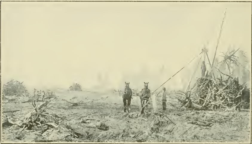
In this operation four men and five horses are used to pile the stumps. The gin-pole is a modification of the swinging boom derrick. The operation is rather expensive owing to its comparative inefficiency compared to hand-handling of the stumps when they are well broken.
