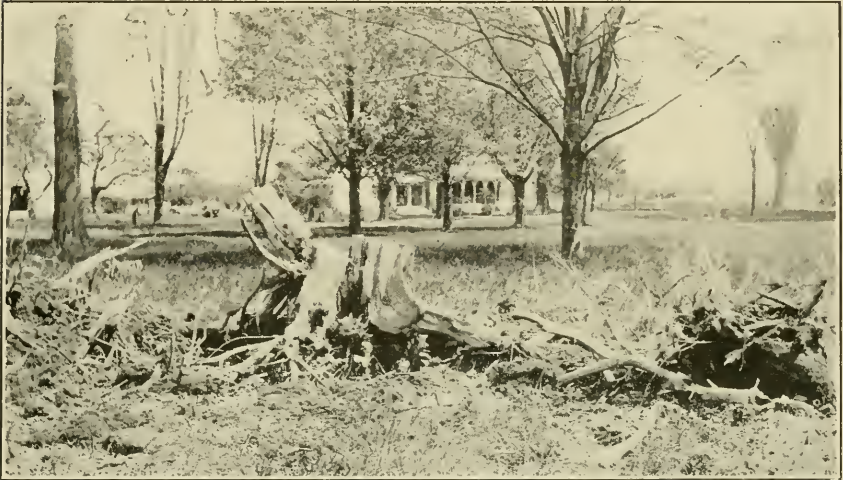
The blaster located his charges under this stump too far toward one side. The result is that the roots of the other side are left sticking in the ground and require another blast.
