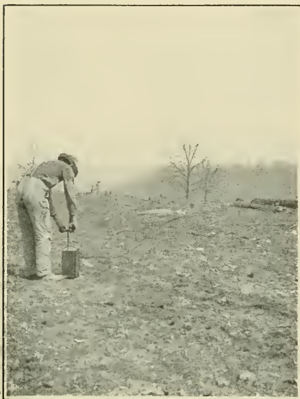
The charges are placed and the wires connected, the stock has been chased away and the helpers warned back—now the blaster is ready to shove the handle of his machine down and to fire the explosive.
