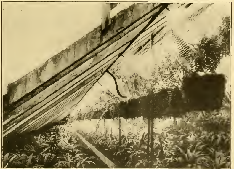
This Cut Shows a Row of Boston Feras being Watered by the Wittbold System. The Same Line of Pipe also Waters Two Benches.
