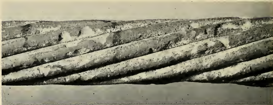
Fig. 15 — Corrosion pockets in galvanized steel armor wires of submarine cable after 12 years of service.
