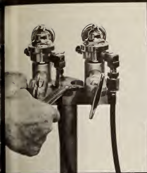
C. Disconnect hose on Oxygen side of yoke assembly on anesthesia unit. It will probably be necessary to loosen with a wrench.
