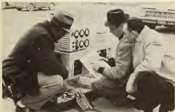
The Chief Building Engineer and two helpers at the PDH operating site carefully examine wiring and operating plan for hospital's generator during Packaged Disaster Hospital training exercise.
