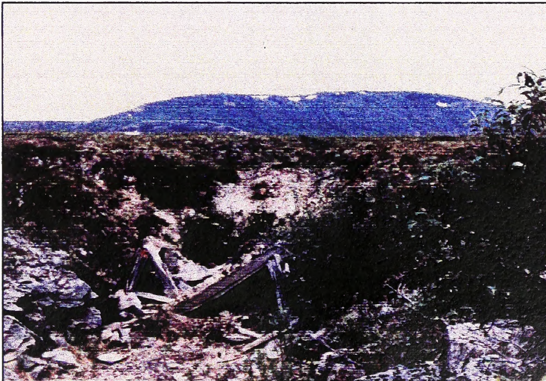
Photograph of lower or western end of the Santa Clara tunnel. Note that timbers are broken and that the near end of tunnel is completely collapsed.
