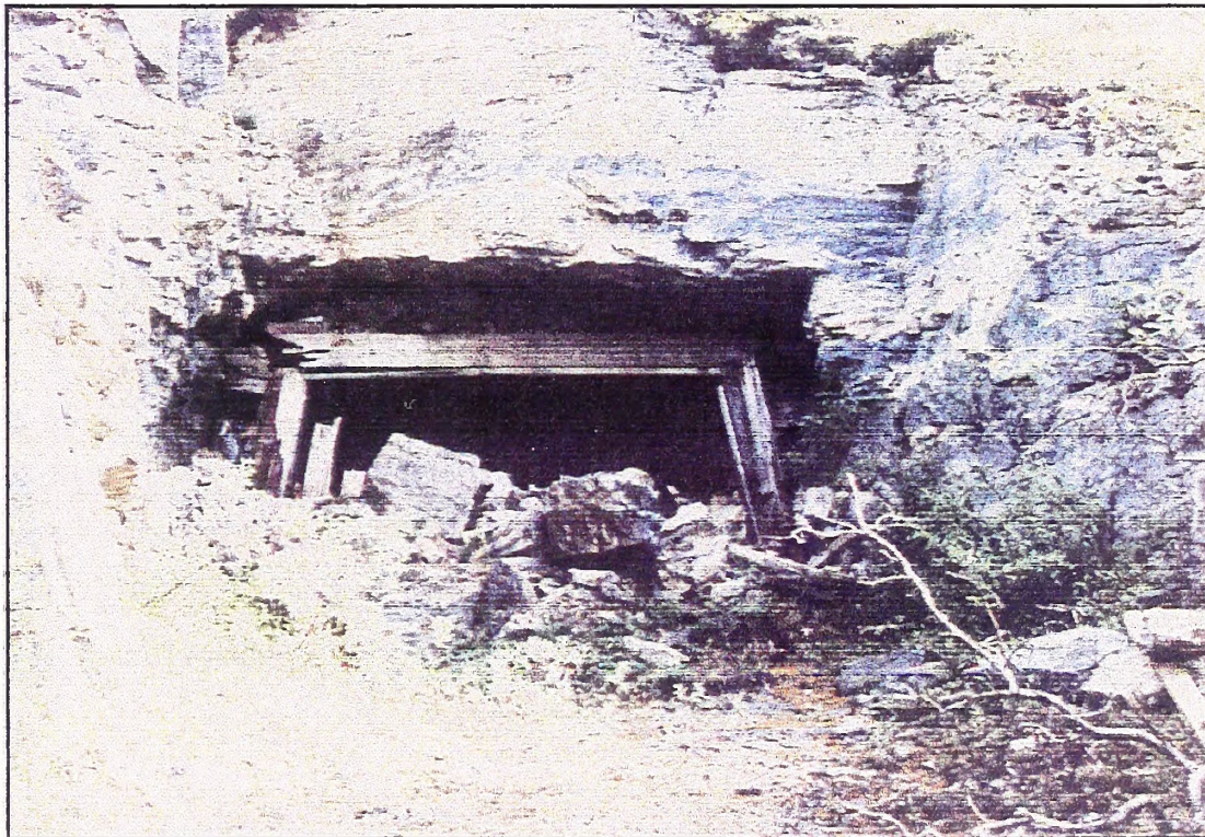
South or lower end of Cape Horn tunnel. This is the least disturbed of any of the tunnel entrances on the Miocene ditch.
