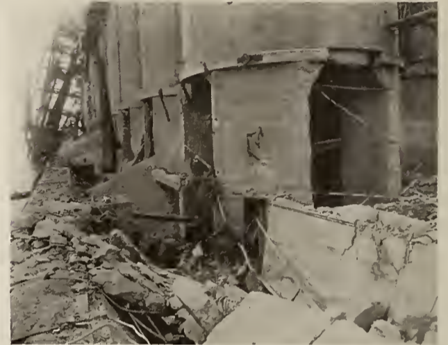
FOUNDATIONS BLOWN OUT FROM UNDER BINS AT NORTH END OF RIVER HOUSE
