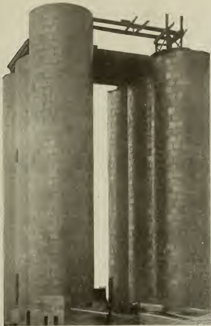
Tile Grain Bins for C. H. Clark Grain Co., Cook's Station, Ohio. Photograph taken during construction.
