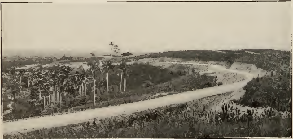
Road Building in Pinar del Rio—View of New Road from Los Mogotes.
