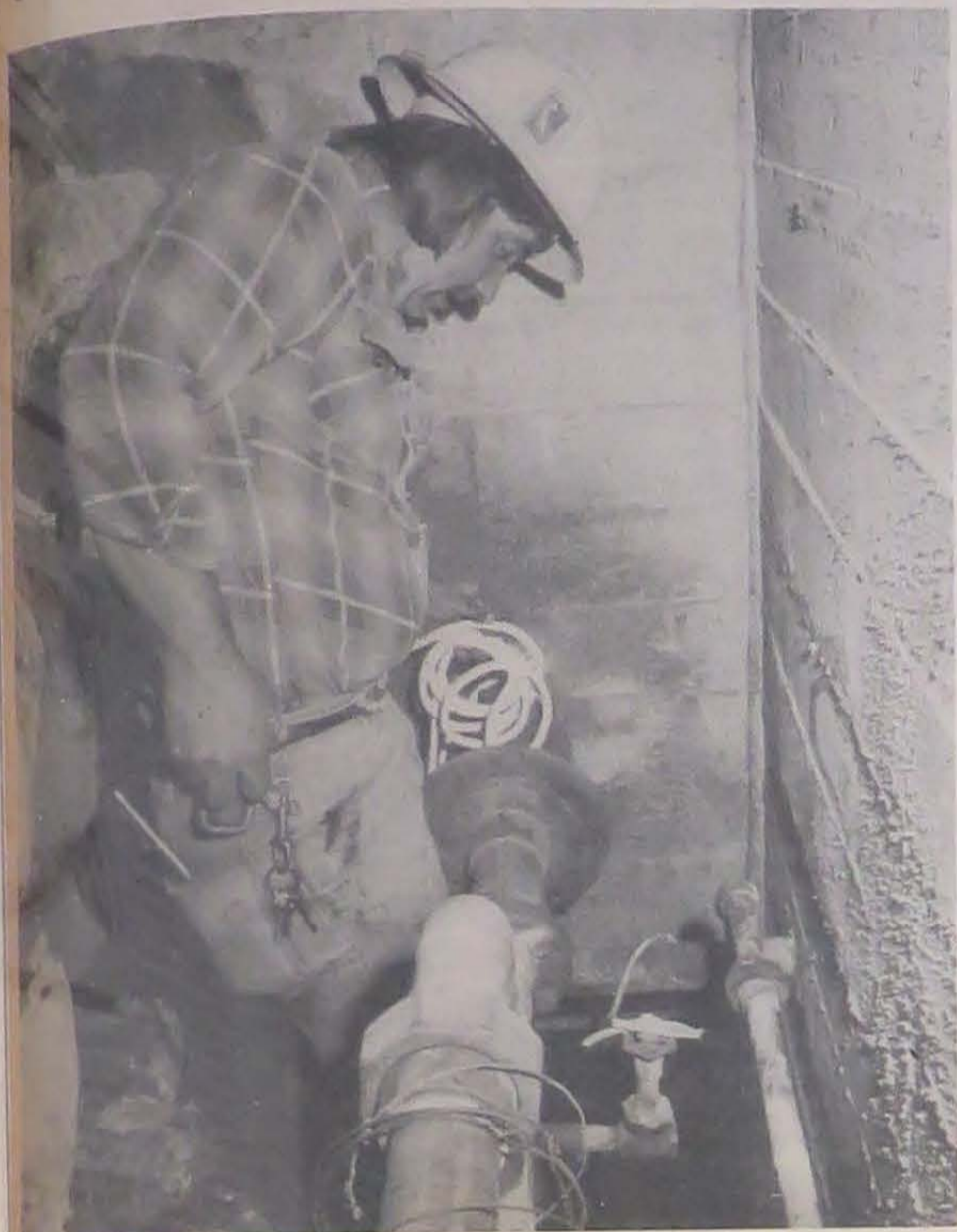
WEEKEND DUTY —PWC Pipefitter Dave Pennock works on Saturday to repair a leak in the steam service provided to the Navy Motel, Barracks, Credit Union, Preventive Medicine School and Alcohol Rehabilitation Service.
