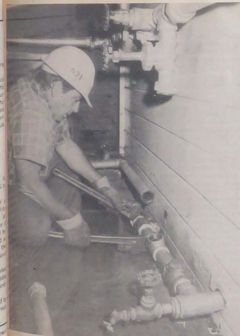
RENEWING THE SYSTEM —PWC Boiler Plant Operator Donald Coons repairs a water pipe inside the boiler plant at Oak Knoll. The work was tied in with the outage during a recent steam leak repair project here.
