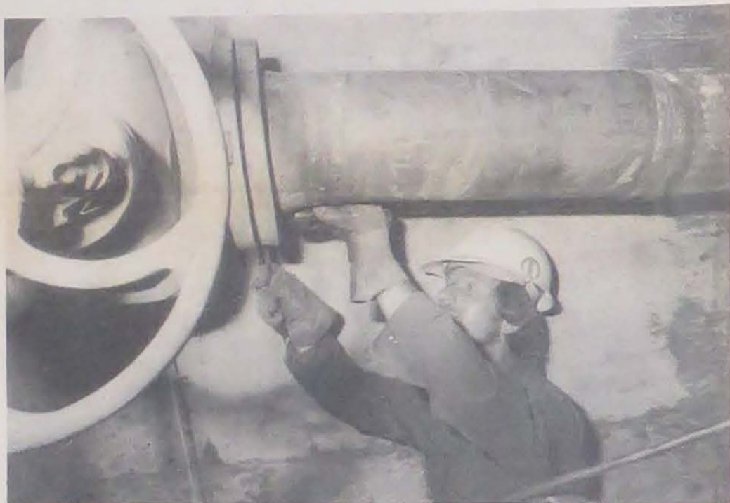
CLOSING IT UP —PWC Pipefitter Mike Debol works on steam leak repair in a manhole behind the main hospital building.
