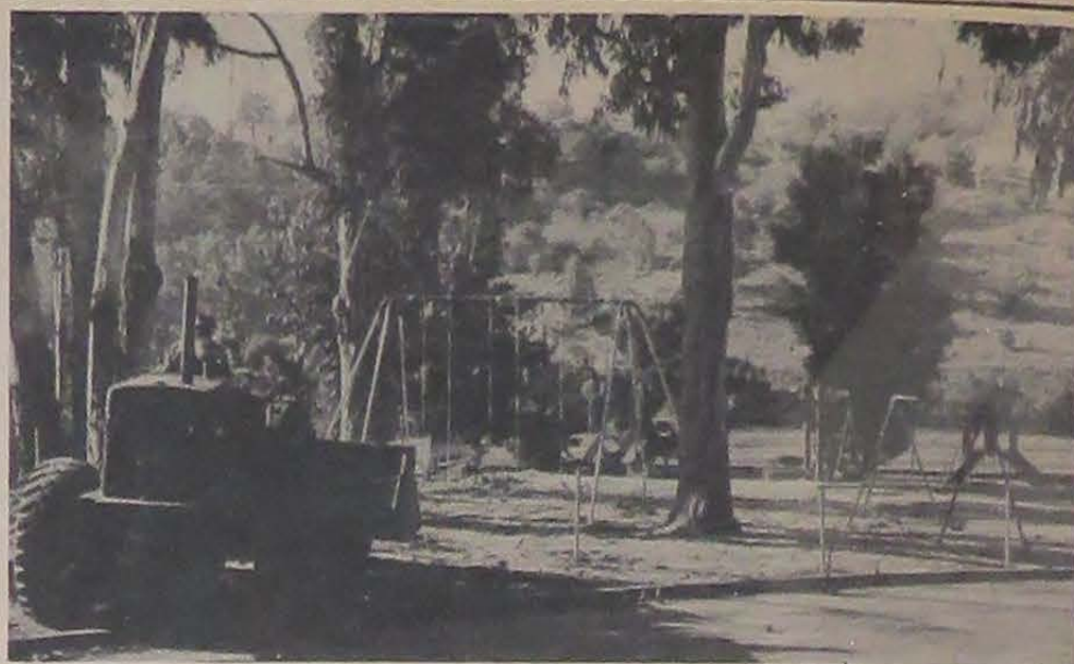
HOW DO YOU PARK THIS THING? —Equipment Operator Constructionman Kevin Cogan does his thing with heavy equipment as he uses a CBU 416 bulldozer to level the earth on the local newly remodeled playground. The new playground equipment includes a conventional swing, a tire swing, various climbing apparatus, and slides.
