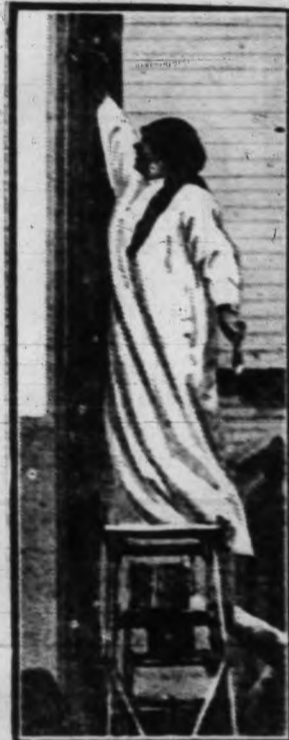
EFFICIENCY. —Members of the congregation of the Ascension Memorial Church of Ipswich, Mass., recently turned out and painted their church building, thereby saving a considerable amount of their treasury fund. Photo shows Mrs. Roger Warner atop a ladder, working busily.
