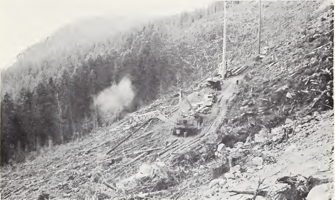
Photo 3.--Cable yarding system operating on steep ground in the Clackamas Subbasin. Mt. Hood N. F. photo. No. 2
