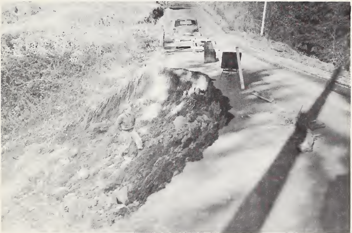
Photo 23.--A road slide is the result of heavy and prolonged rains and floodwaters, subbasin 8. SCS photo. 7-597-11
