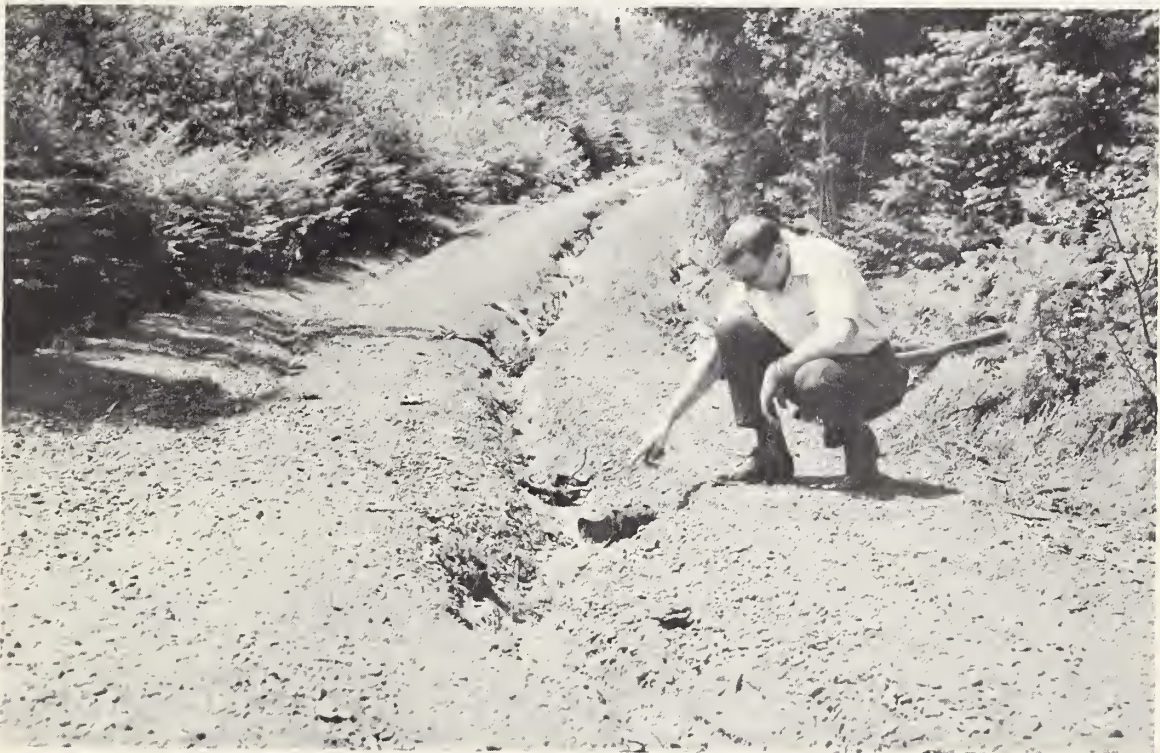
Photo 35.--Inadequate ditches and cross drains cause this type of erosion on forest roads. Note small broken cross drain. Survey Party photo. 7-1397-4
